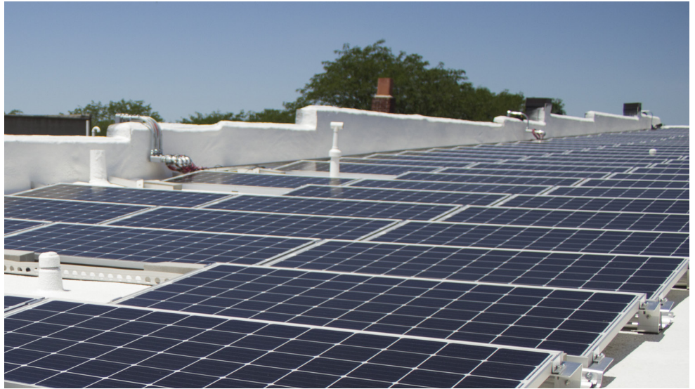
A rooftop solar array in Norfolk. While some homes and commercial buildings can have their own solar arrays, community solar projects provide an opportunity for others in a village or city to benefit from solar energy.
