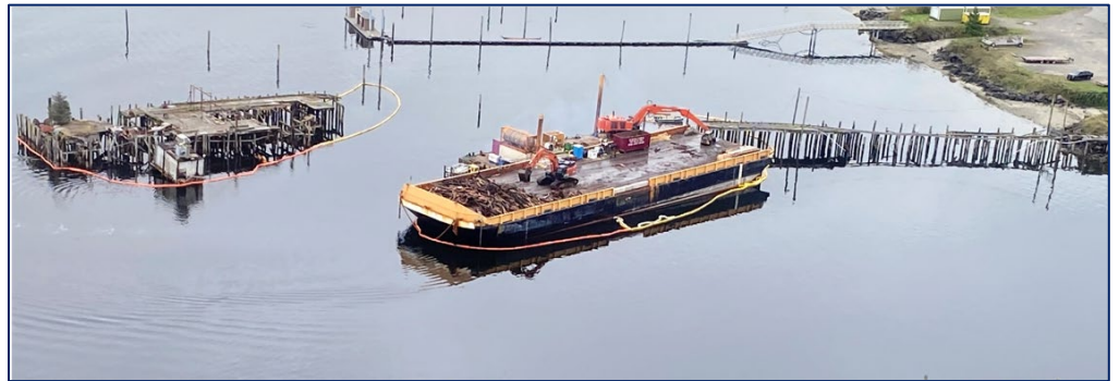
Deconstruction of the Former High Tides Seafood Pier in Neah Bay, WA
