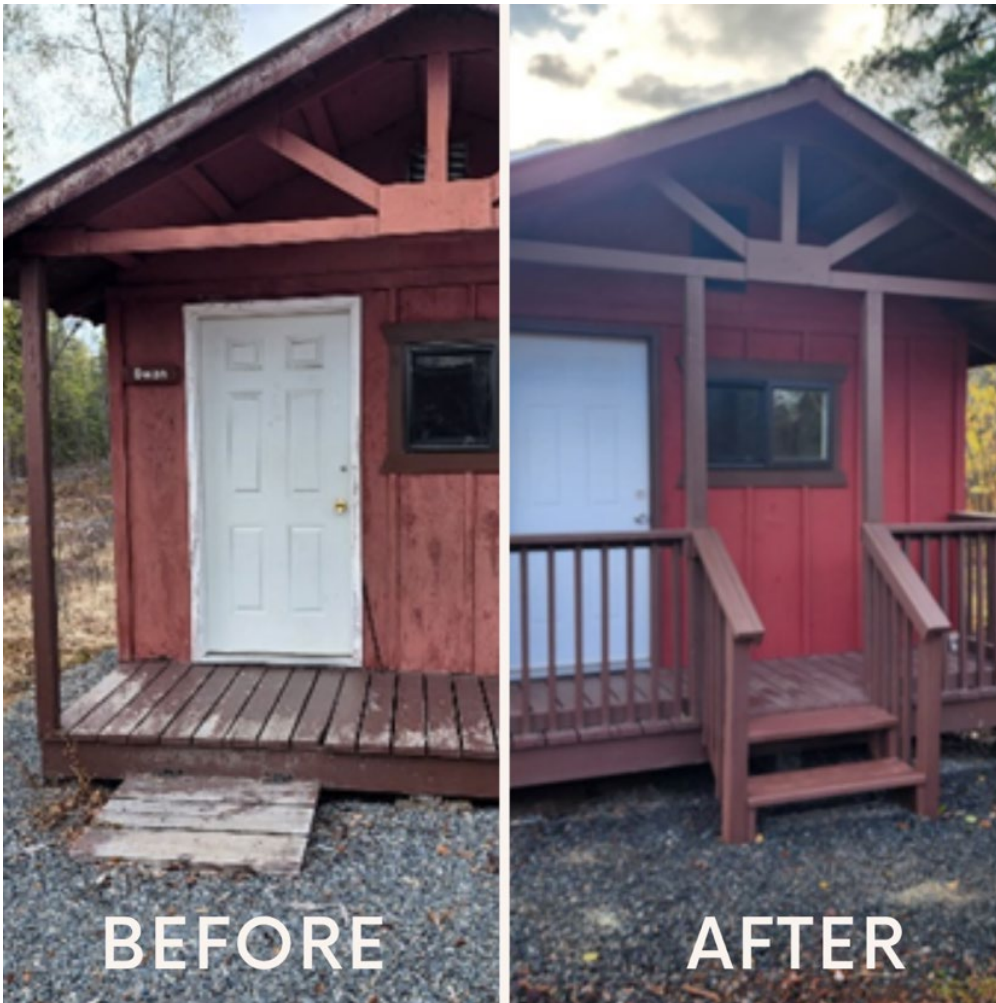
Rehabilitation of six cabins at Kenai NWR in Alaska by NWRS maintenance professionals saved the Service over $166,000 compared to traditional contracting costs. Completed in December 2023.
