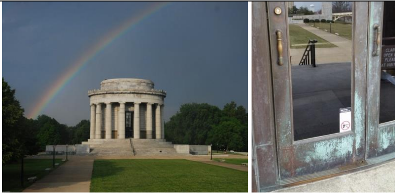
Left: Memorial Building Right: Corrosion of Bronze Doors
