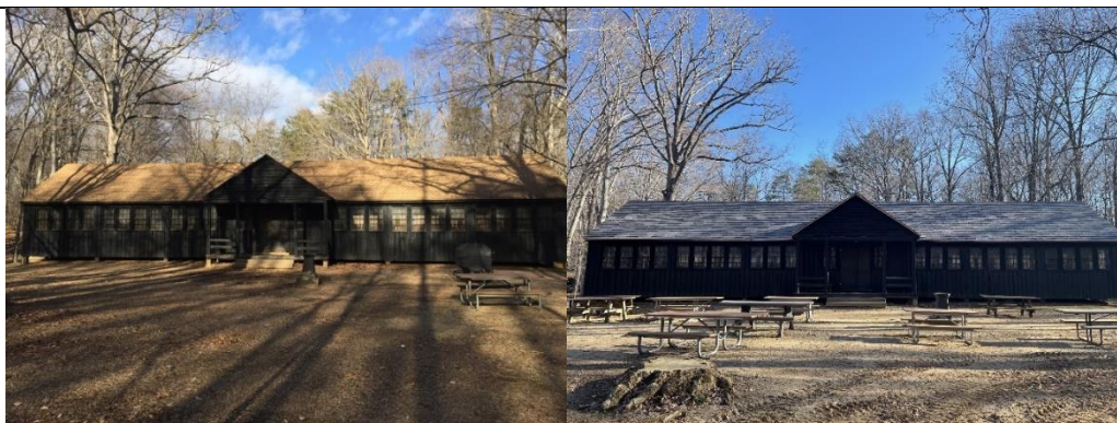
Left: The deteriorated asphalt shingle roof, contrasting with the building's décor. Right: The replaced roof, with added weather shielding and more appropriate aesthetics.
