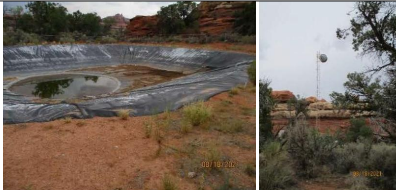
Left: Evaporation pond at Needles water treatment plant.
