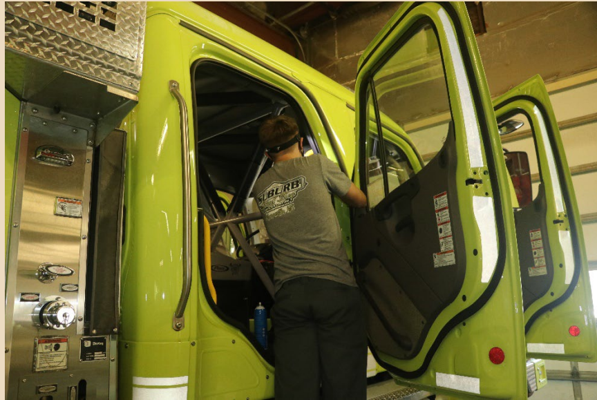
Installation of a roll cage in a BLM wildland fire engine at NIFC in Boise, Idaho. (Photo by BLM.)
