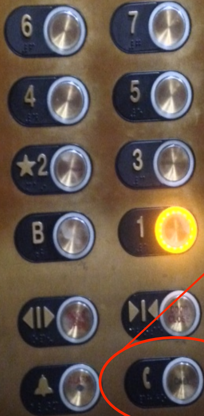
Left Side Control Panel
