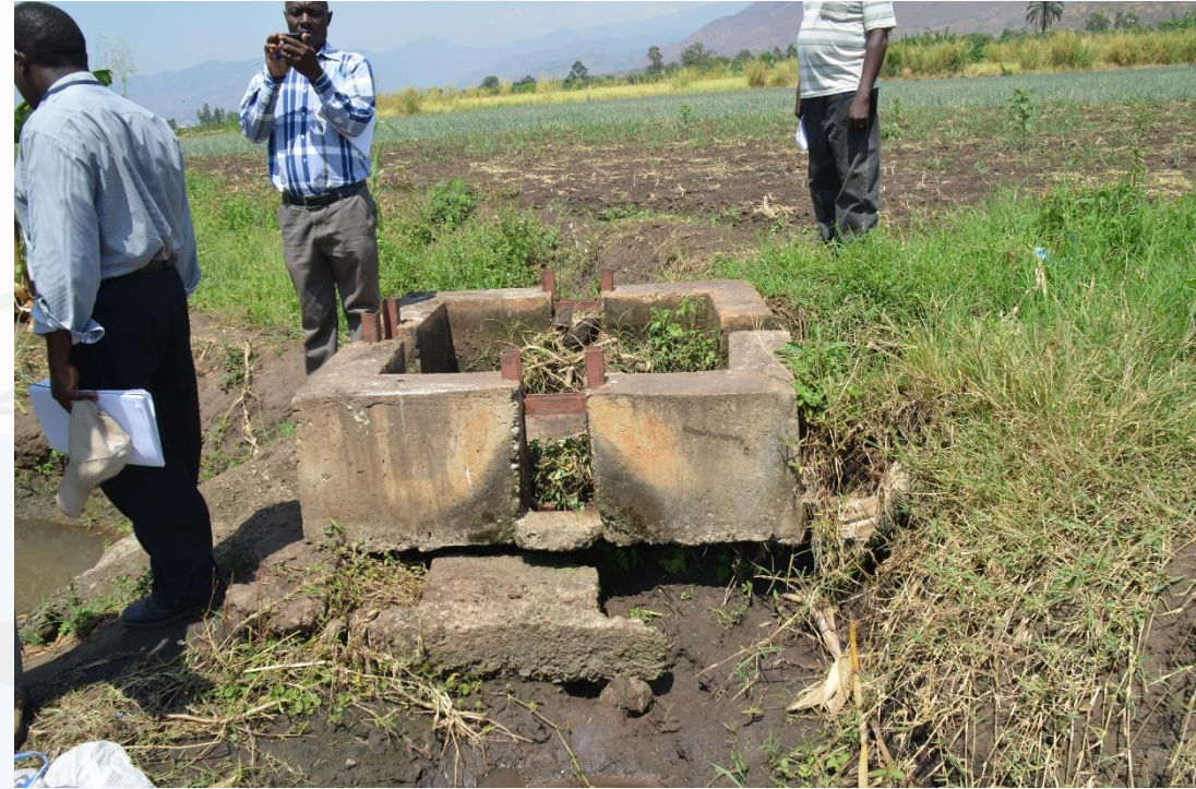
Fig.3: Dilapidated tertiary canal & turnout
