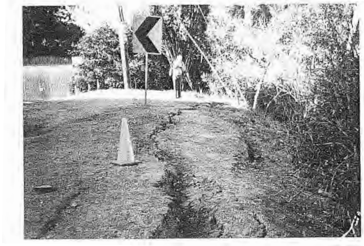
Figure 7-4 Slope Failure with Ground Cracking along Mulholland Drive, 1994 Northridge Earthquake (after EERI, 1995)
