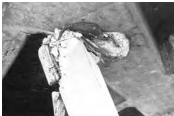
Figure 1-11 Shear Failure of the Head of a Pile at the Struve Slough Bridge
