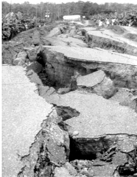
Figure 7-10 Disrupted Fill and Pavement due to Liquefaction at the Approach to the Highway 36 bridge Over Rio Estrella, Costa Rica, during 1991 Earthquake.
