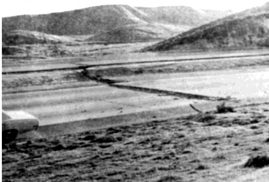
Figure 7-6 Differential Settlement across Pavement Joints Near Cut-fill Boundary on I-5 north of I-405 Separation. The Settlement is due to Seismic Compaction of Fill during the 1971 San Fernando Earthquake.
