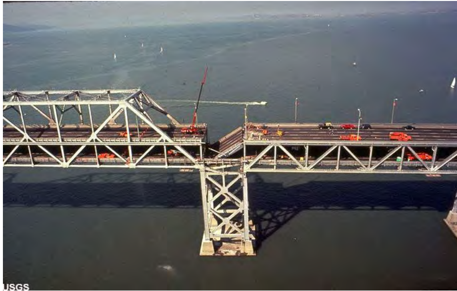
Figure 1-7 Damage to the San Francisco-Oakland Bay Bridge East Span due to the 1989 Loma Prieta Earthquake (USGS)
