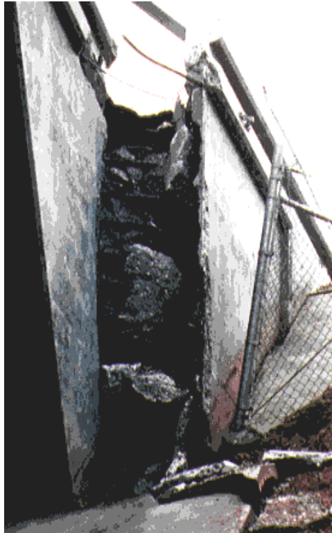
Figure 1-8 Failure of the Wingwall at the Roxford Street Undercrossing in the 1971 San Fernando Earthquake
