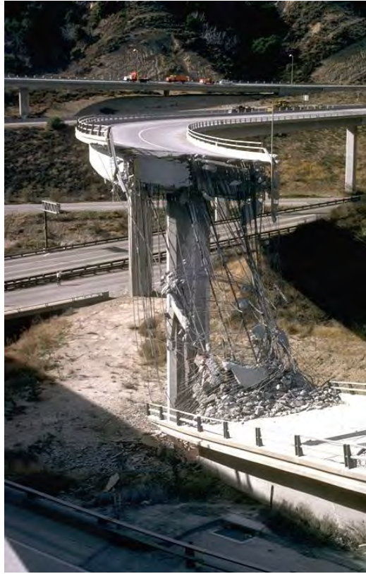
Figure 1-13 Collapse of the I-5, SR-14 Interchange in the 1994 Northridge Earthquake (USGS)
