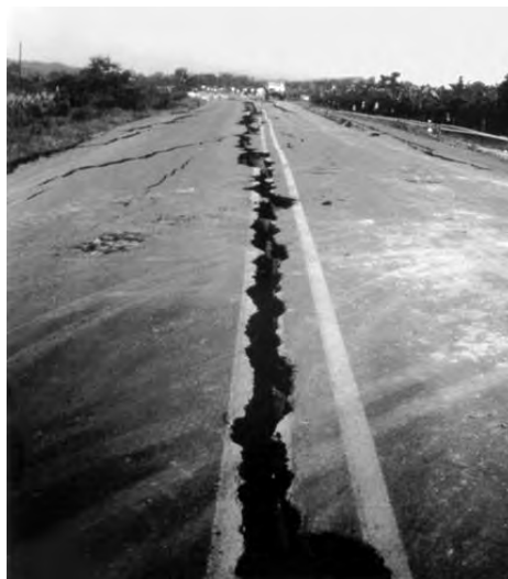
Figure 7-9 Segment of Highway 36 Near Caribbean Coast in Costa Rica that Split Longitudinally, Settled and Spread Laterally during 1991 Earthquake by Mechanism
