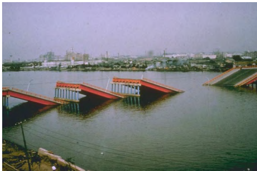
Figure 1-5 Collapse of the Showa Bridge in the 1964 Niigata, Japan Earthquake (NGDC)
