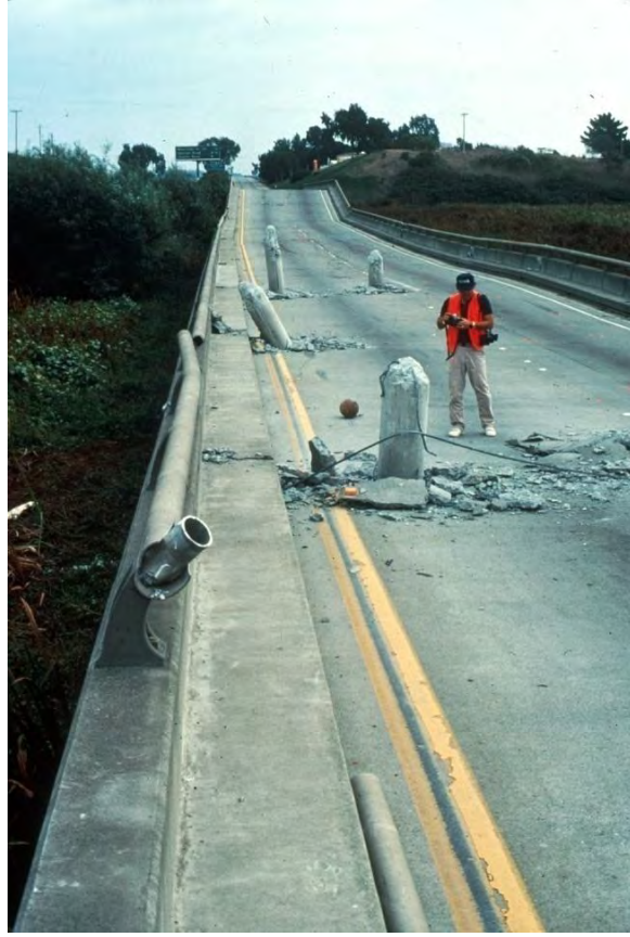
Figure 1-10 Collapse of the Bridge over Struve Slough in the 1989 Loma Prieta Earthquake (USGS)
