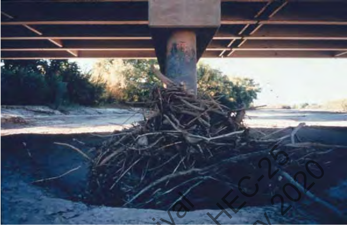
Figure 9.5. Scour at a Coastal Bridge Pier
