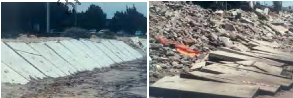
Figure 6.14. Example of a failed attempt at embankment protection (USACE archives photo)
