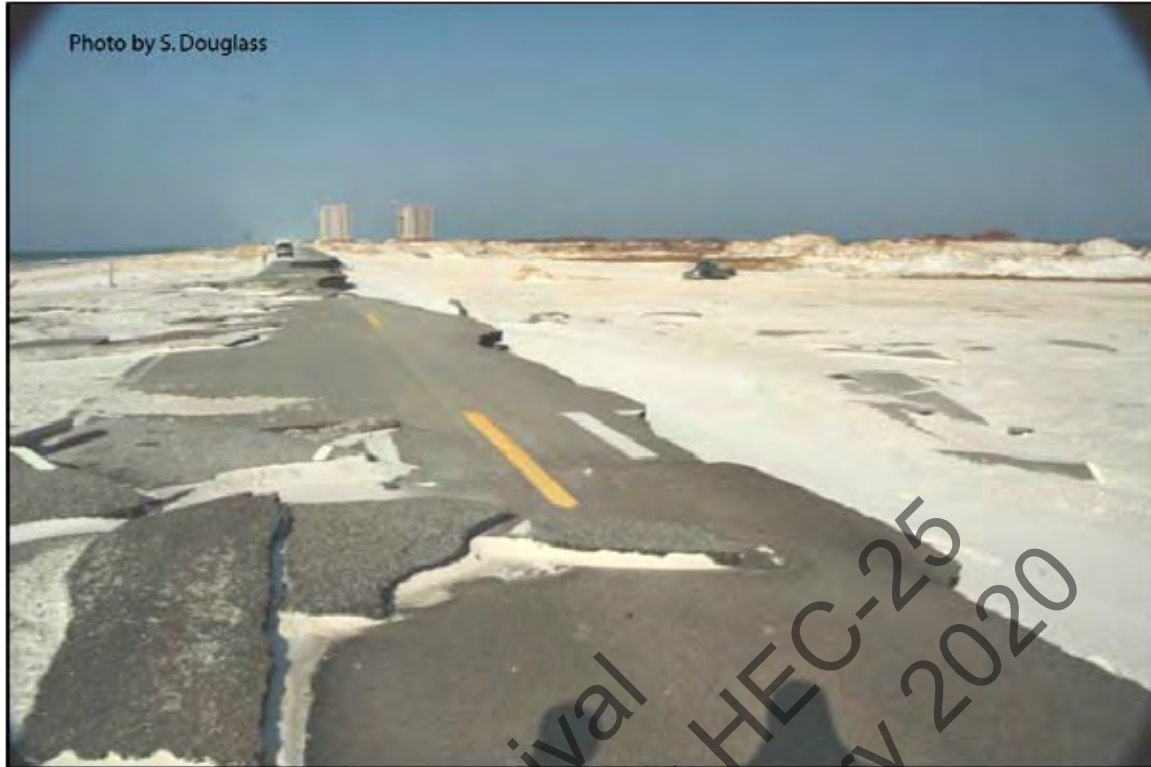
Figure 8.3. Example of pavement damaged by Hurricane Ivan. (photo looking west on Florida 399, J. Earle Bowden Way, Gulf Islands National Seashore, September 2005)
