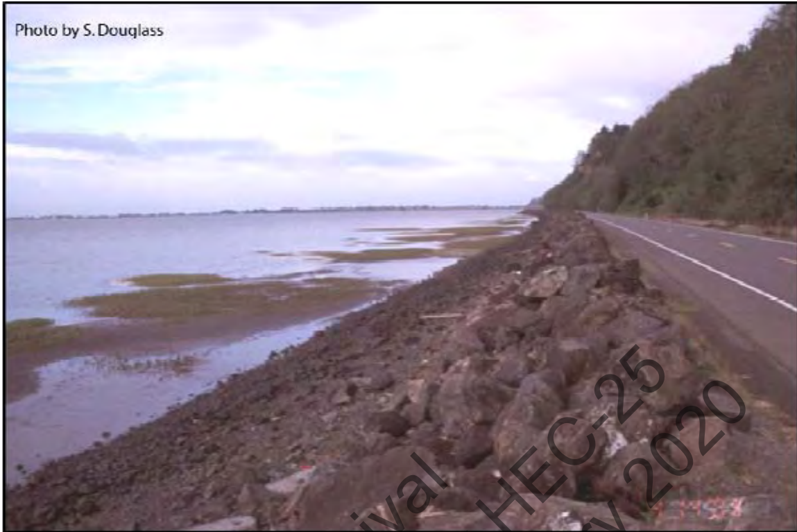
Figure 6.10. Revetment protecting a highway along a bay shoreline. Washington State Route 105, Willapa Bay, Washington (2003)
