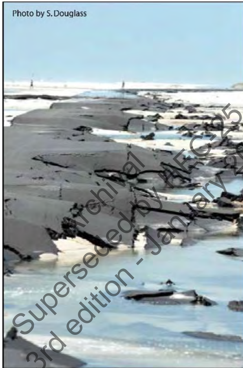
Figure 8.6. Pavement destroyed by the weir-flow mechanism (Ft. Pickens Road, Gulf Islands National Seashore, near Pensacola, Florida).
