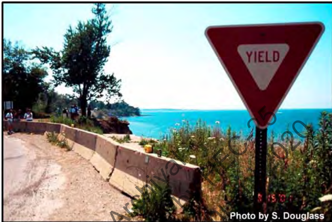
Figure 7.4. A local road being undermined by bluff erosion and long-term shoreline recession on the Great Lakes. Painesville, Ohio (2001)
