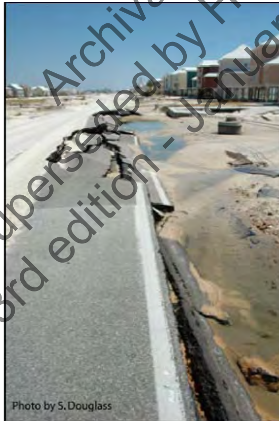
Figure 8.15. Evidence of weir-flow damage to the seaward edge of pavement due to return flow late in the storm (West Beach Blvd., Alabama 182, Hurricane Ivan, Gulf Shores, Alabama).
