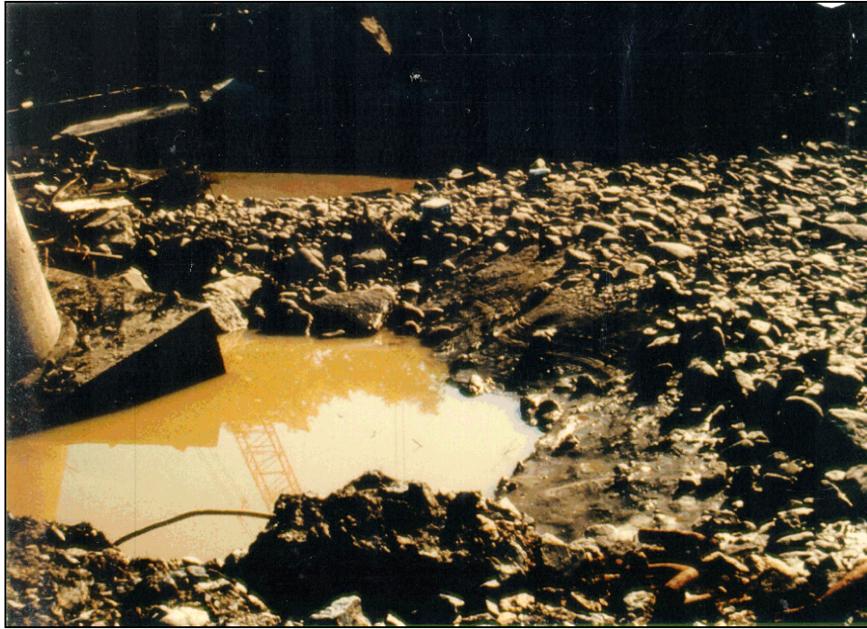
Figure 5.17. Pier scour holes at Schoharie Creek Bridge in 1987. Pier 2 in the foreground with pier 3 in the background.
