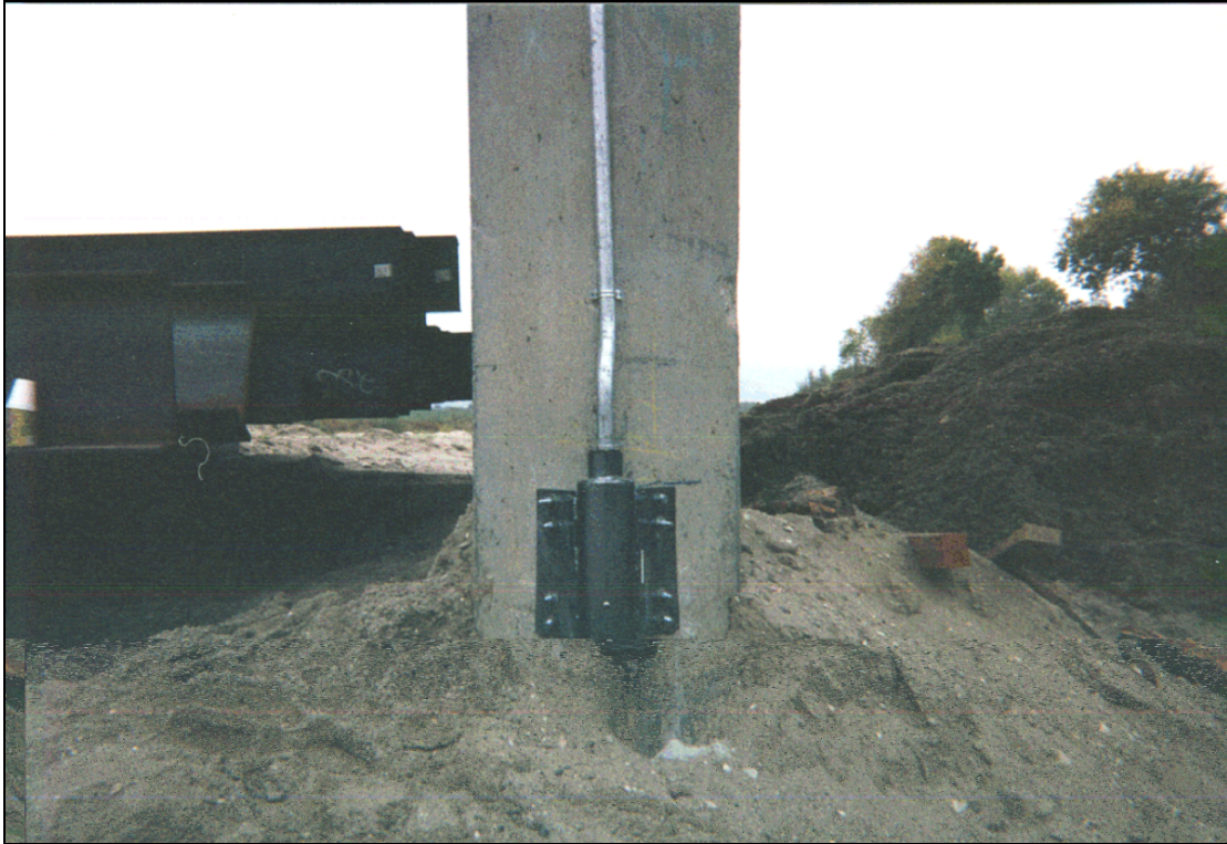
Figure 9.28. Close up of sonar scour monitor on Salinas River Bridge near Soledad, CA.
