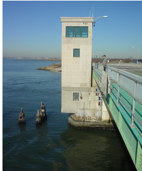
Figure 9.24. Conduit to sonar scour monitor at Wantagh Parkway over Goose Creek.
