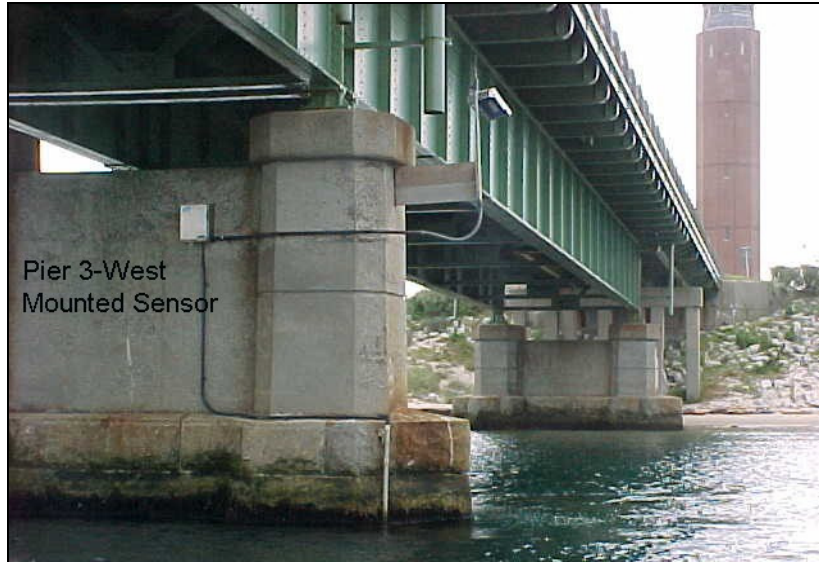
Figure 9.13. Sonar scour monitor installation including remote station and solar panel.
