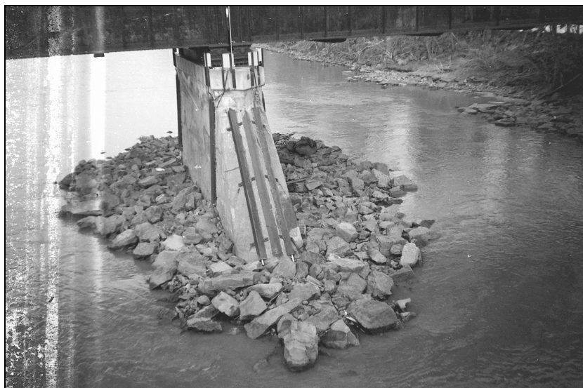
Figure 9.21. Brisco Monitor sounding rods installed at a bridge pier in New York to monitor movement of riprap (Butch 1996).
