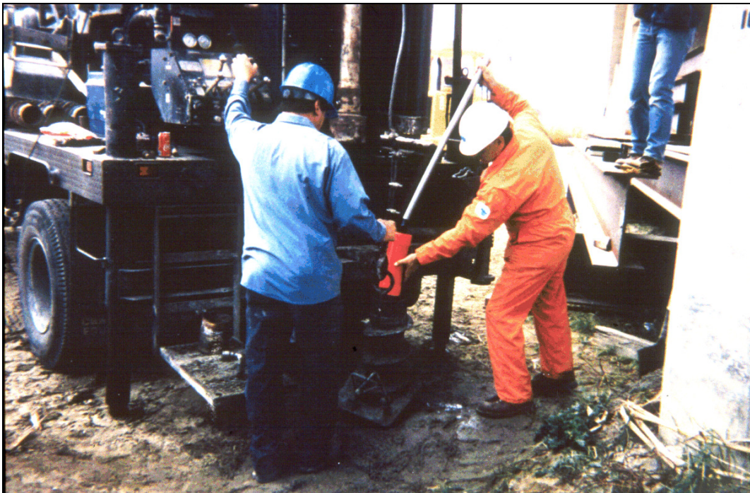
Figure 9.30. Installation of float out device on Salinas River Bridge near Soledad, CA.
