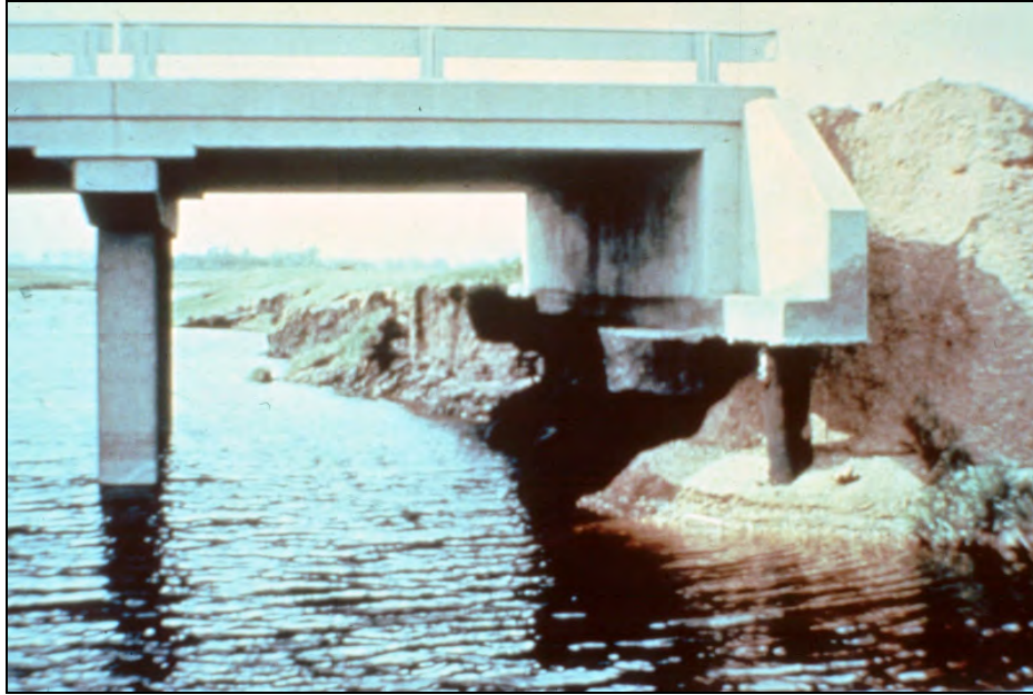
Figure 14.1. Scour of bridge abutment and approach embankment.
