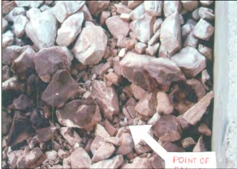
Figure 5.9. Riprap failure in 1997 tests ( d_{50} = 0.89 ft (271 mm)).
