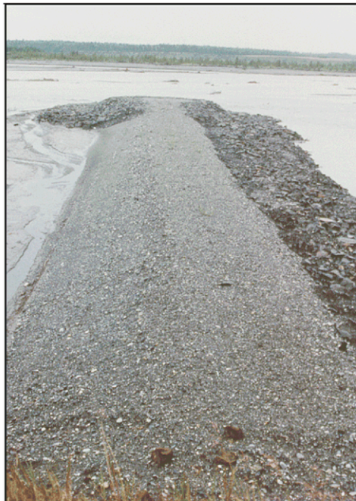
Figure 2.13. Impermeable spur field in top photograph with close-up shot of one spur in the lower photograph, vicinity of the Richardson Highway, Delta River, Alaska.
