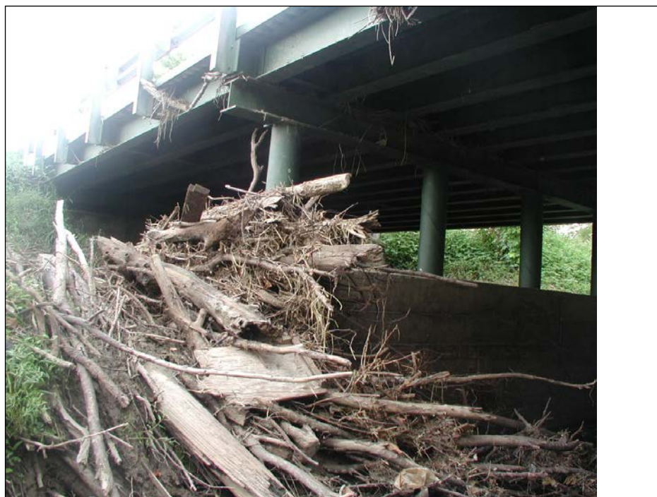
Figure 7.15. Woody debris at a bridge pier. Note how debris can be much wider than the pier itself (also note debris on lower chord of bridge deck). Source: NCHRP Web-Only Document 48 (see NCHRP 2010a).
