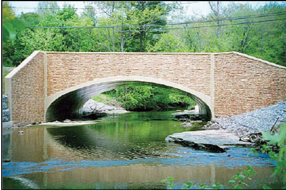
Figure 6.13. Open-bottom culvert on Whitehall Road over Euclid Creek in Cuyahoga County, OH.
