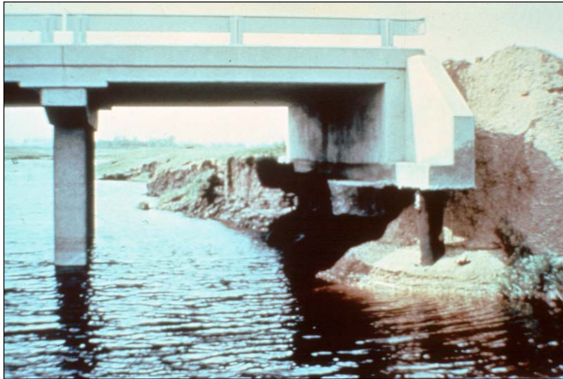
Figure 8.2. Scour of bridge abutment and approach embankment.
