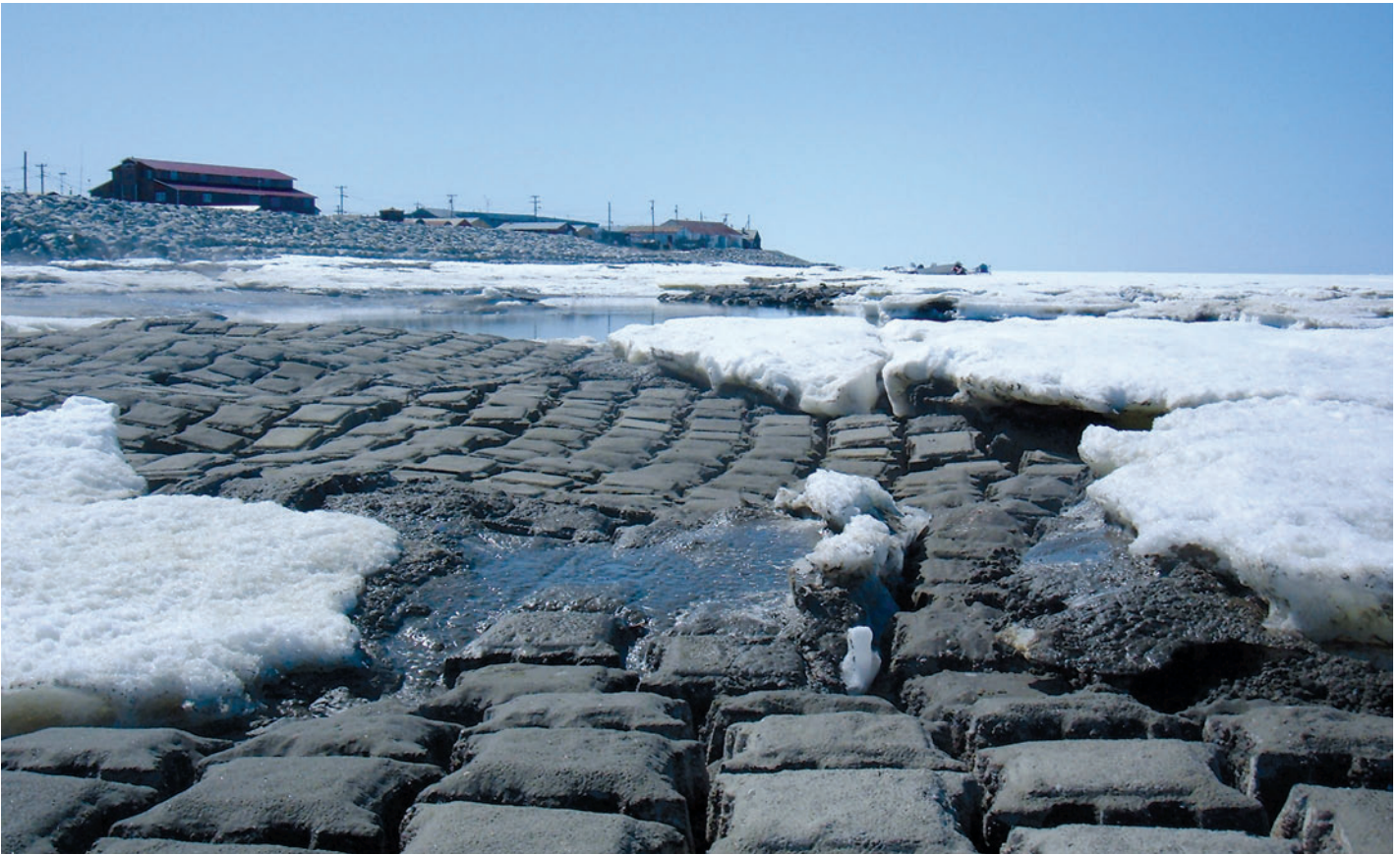
Figure 3: Melting Sea Ice Reveals Prior Control Efforts and the Advance of Erosion toward the Seawall Being Constructed in the Village of Shishmaref, Alaska, June 2008
