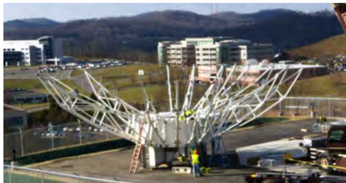
Above: Antenna construction at the RBU in Fairmont, WV: Site 3 Reflector Assembly
