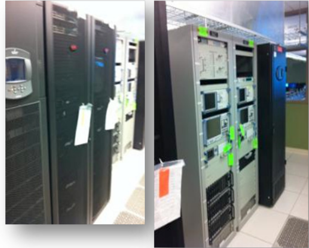
EI installation at RBU. Credit: Harris Corporation
