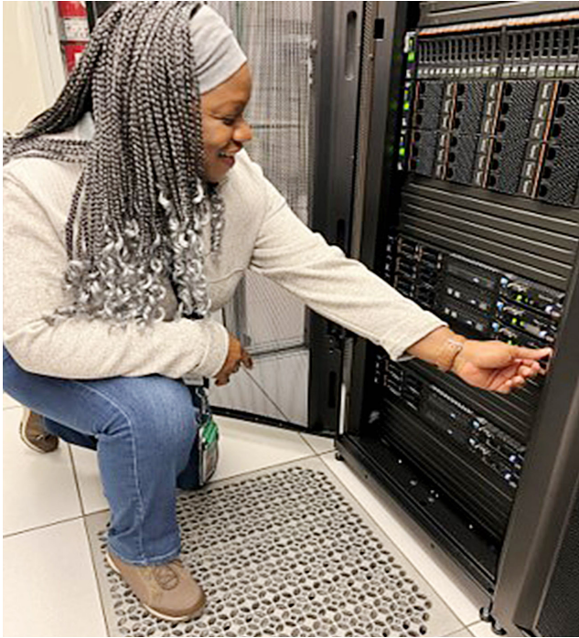
An L3Harris team member tests new server equipment at the Consolidated Backup. Photo credit: L3Harris
