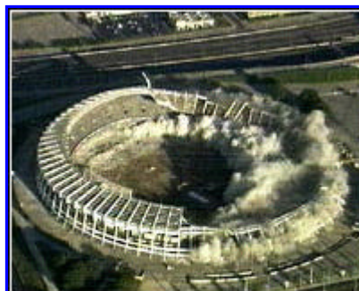
Like a set of dominoes, the former home of the Atlanta Braves collapsed
