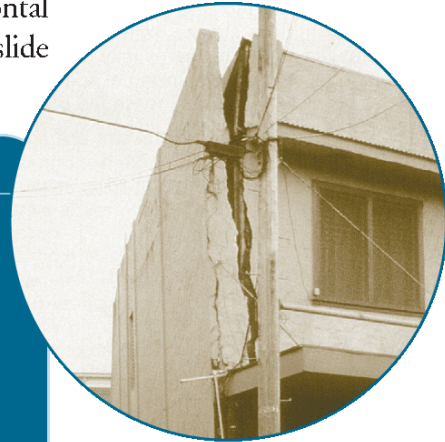
Hilo building damaged by the November 1983 Kaoiki earthquake.
