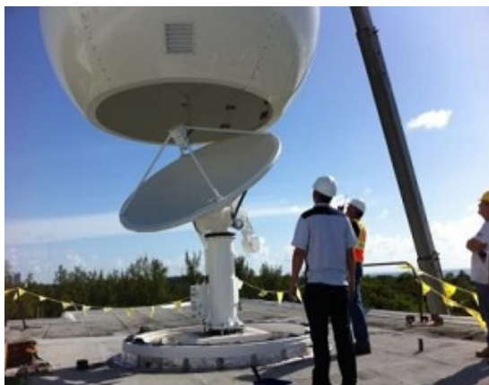
The full direct broadcast antenna network covers all of North America and provides reliable data to NOAA's National Center for Environmental Prediction to assist in meeting the nation's environmental challenges while also allowing local markets to collect data directly from Suomi NPP.
