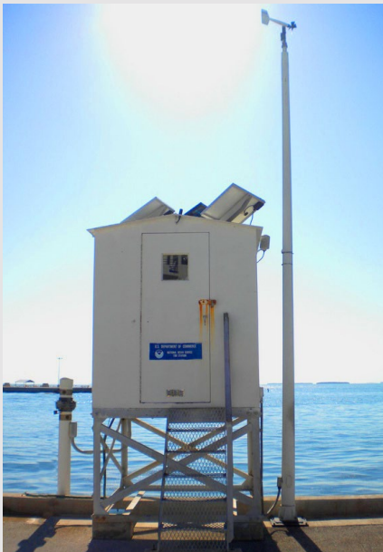
Tide gauge station in Key West, FL. Credit: NOAA/NOS
