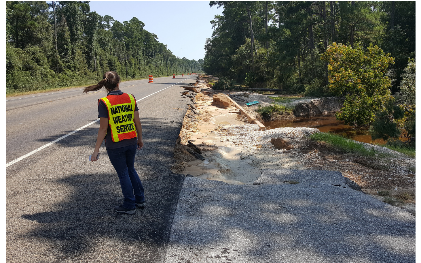
Meteorologists from NWS Houston survey flood damage following Hurricane Harvey.
