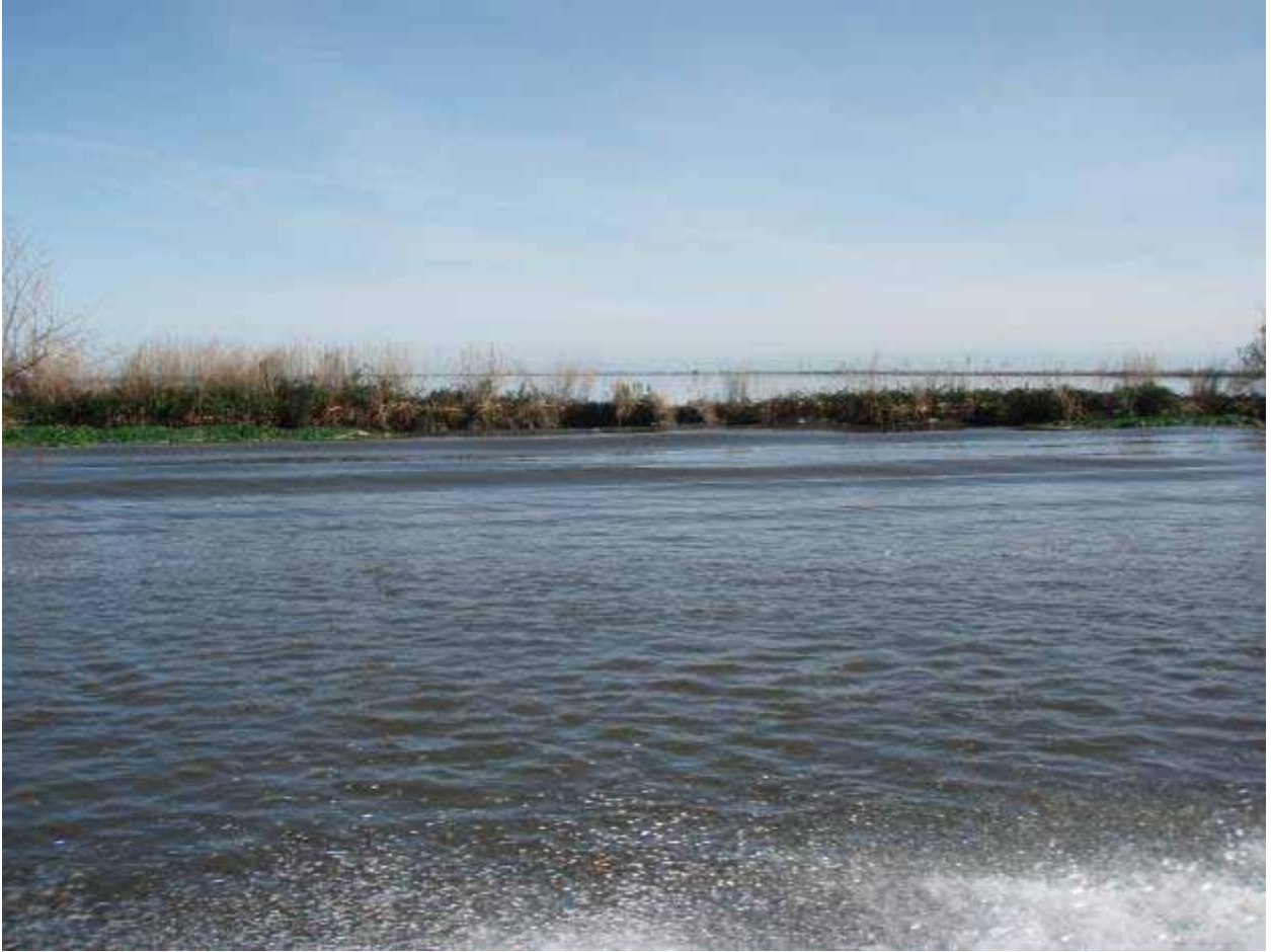
Figure C-6 - Mildred Island, showing effect of flooding on levee
