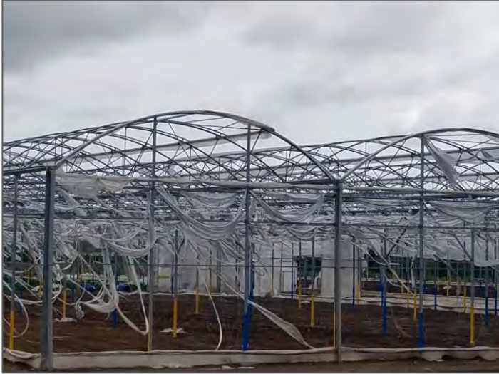
damaged infrastructure after a wind event
