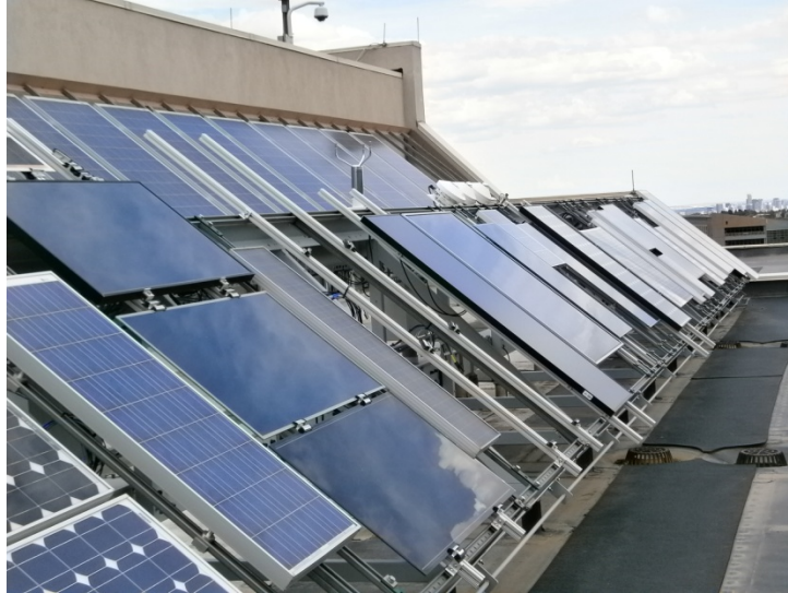
Figure 2-3. PV modules deployed on the PERT at NREL, Golden, Colorado
