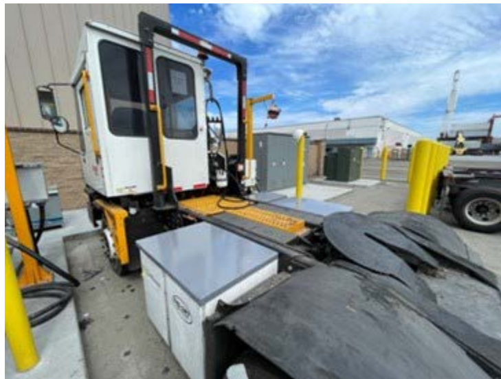
Figure 30. Electric Yard Tractors with Battery Pack Protection Covers
