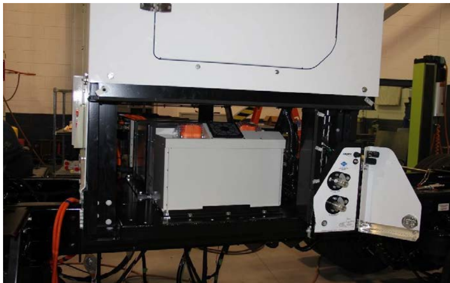
Figure 8. High-Voltage Battery Integrated into Hydrogen Storage Cabinet
