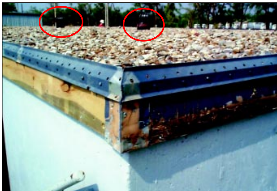
FIGURE 6-14: Ballast roof covering on a community shelter in Wichita, Kansas was a potential source of deadly windborne missiles to those seeking to access the shelter. Circles identify covers protecting roof penetrations intended for ventilation, but unable to provide adequate resistance to windborne debris.
