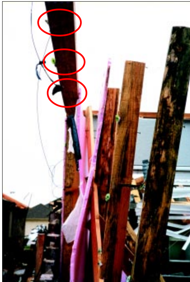
FIGURE 4-9: Failures of the connection of the double-top-plate to the supporting studs below at a home in Moore, Oklahoma. This home was located along the periphery of a violent tornado.
