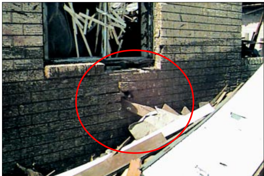
FIGURE 3-19: A 2-in by 6-in missile can be seen completely penetrating the brick veneer of a home in Moore, Oklahoma.
