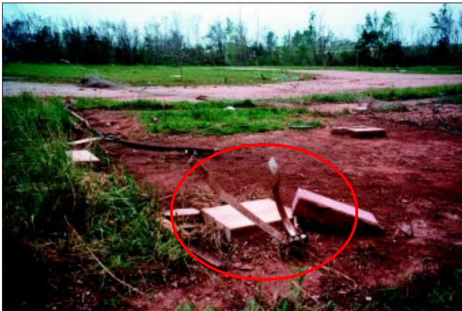
FIGURE 4-48: Failed straps at the anchorage of a manufactured home in Bridge Creek, Oklahoma. This site was 300-400 feet from a violent tornado vortex.
