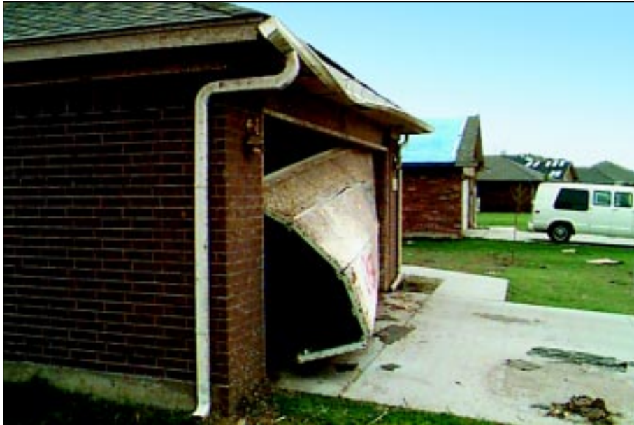
FIGURE 4-18: This double-width garage door failed under a suction load in Moore, Oklahoma.
