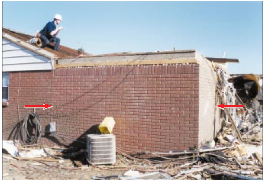
FIGURE 6-1: Aboveground in-residence shelter hit by strong inflow winds near the vortex of a violent tornado in Del City, Oklahoma. Arrows indicate the extent of this reinforced concrete shelter that cannot be seen due to the brick veneer.
