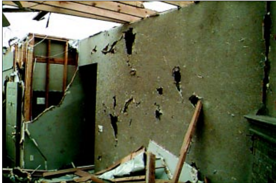
FIGURE 3-30: Several missiles struck and perforated the interior wall of this house in Moore, Oklahoma.
