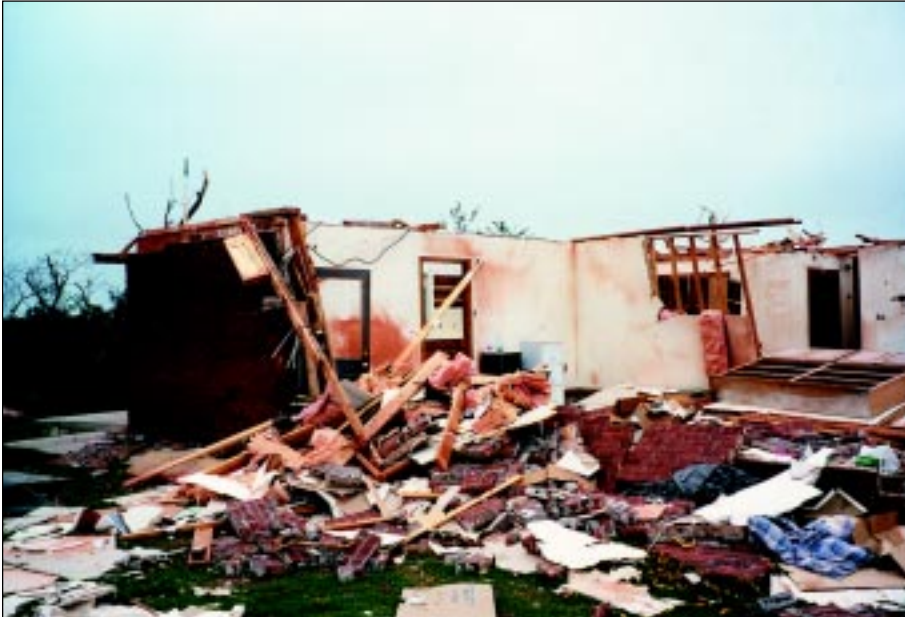
FIGURE 4-32: Failure of brick masonry veneer construction. The vortex of the strong tornado that caused the winds at this site passed approximately 300 feet from this building in Bridge Creek, Oklahoma.
