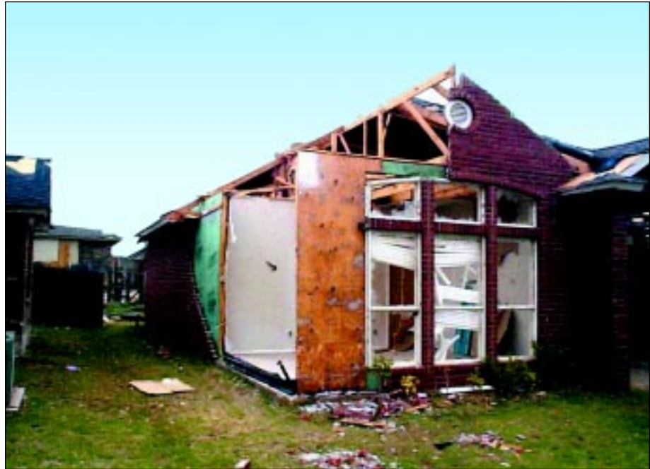
FIGURE 3-9: Failure of this exterior wall and roof section in Moore, Oklahoma, occurred when the windows broke and the front room saw a rapid increase in internal pressure. Most of the debris from the roof and exterior wall had been cleaned up prior to this photograph. This home was located on the periphery of a violent tornado track.
