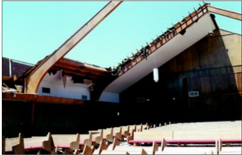
FIGURE 5-10: This church suffered loss of roof due to lack of load path between the rigid laminated wood arches and the roof purlins (missing in photo) that supported roof sheathing. Inflow area of a violent tornado, Moore, Oklahoma.
