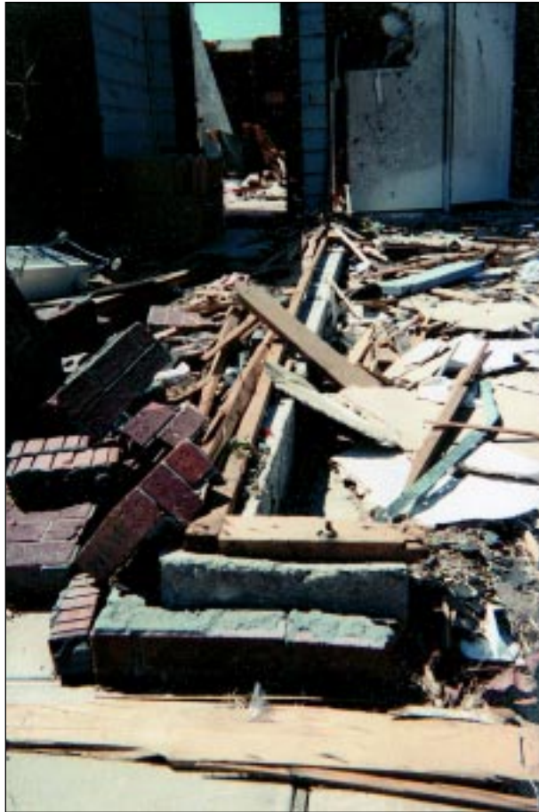
FIGURE 4-13: Failure of this bottom plate to wall stud connection occurred at this home outside Oklahoma City, Oklahoma. The vortex of a violent tornado passed very close to this home.
