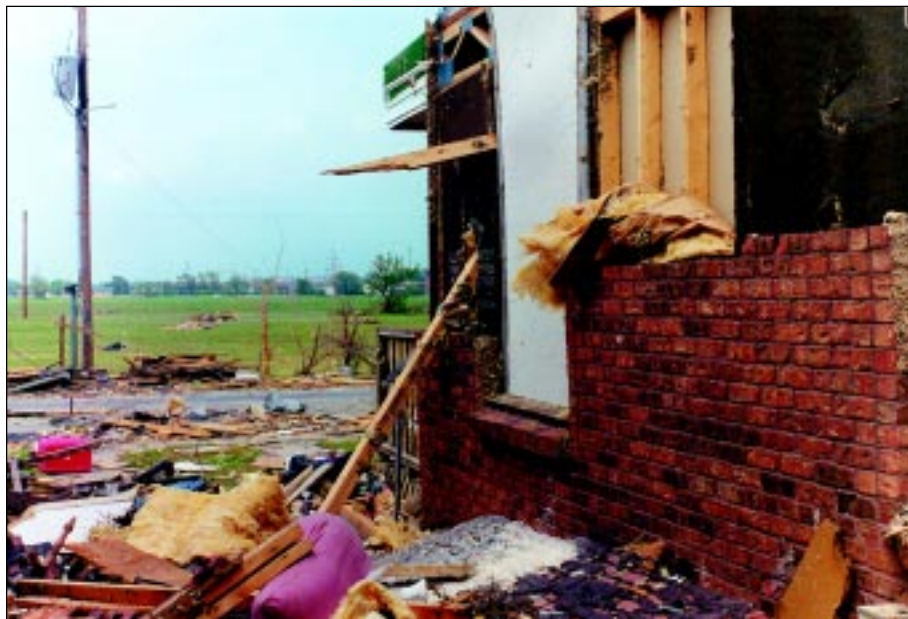
FIGURE 4-45: Failure of brick veneer at a multi-family housing unit in Wichita, Kansas. This building experienced inflow winds from a strong tornado.
