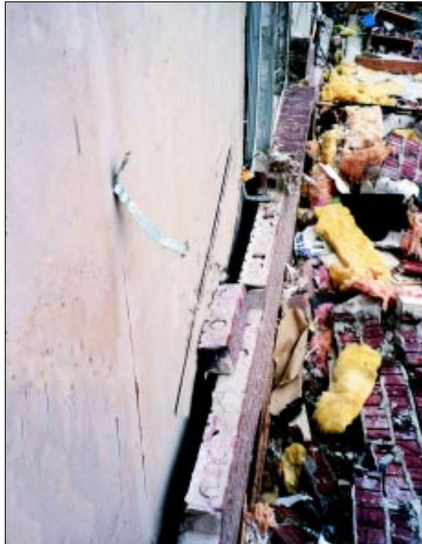
FIGURE 4-36: Inadequate bonding of mortar to galvanized brick ties, Bridge Creek, Oklahoma.
