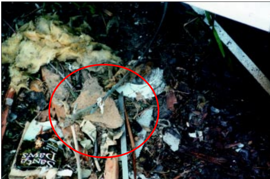
FIGURE 4-52: Strap torn off from chassis of manufactured home. This home in Wichita, Kansas, was located within the inflow area of a strong tornado.
