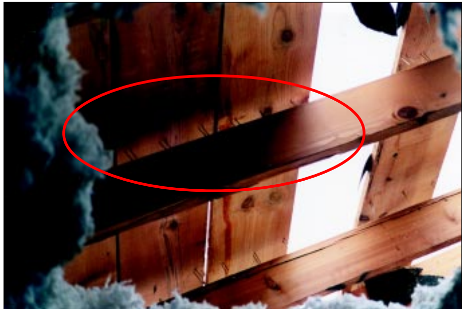
FIGURE 4-3: Failed stapling of boards to rafters viewed from home in Moore, Oklahoma.
