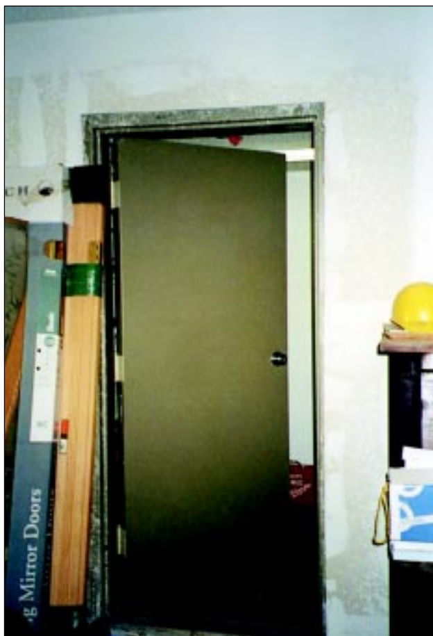
FIGURE 6-3: Entrance to the ICF shelter in Bridge Creek, Oklahoma. This residence and shelter were on the periphery of the inflow winds of a strong tornado, and damage was limited to light missile impacts.
