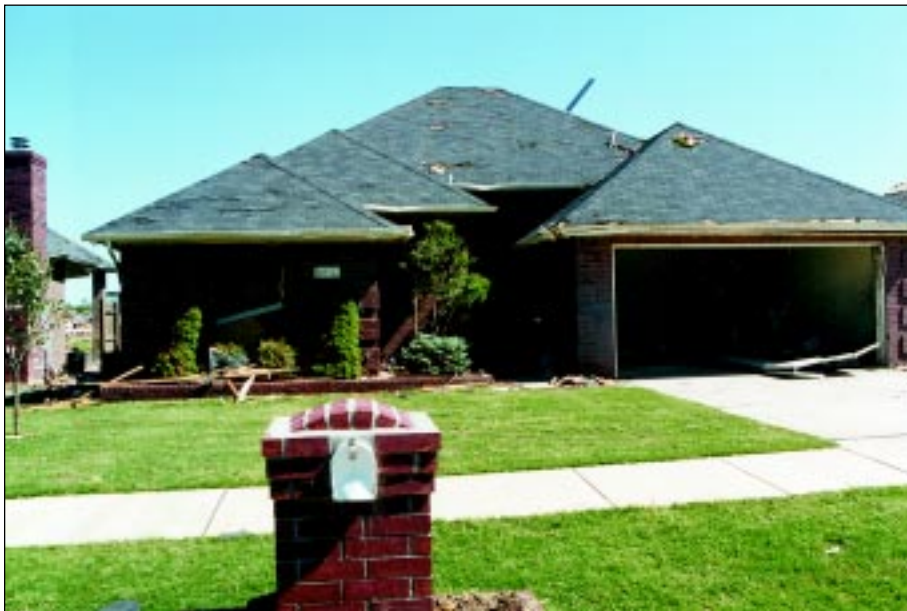
FIGURE 4-24: A view of home G with a garage door that failed due to positive (inward) acting wind loads.
