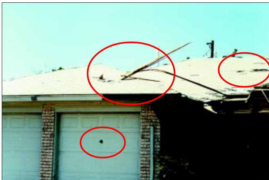
FIGURE 3-28: This house was on the periphery of a violent tornado damage area in Moore, Oklahoma. Two medium missiles are embedded this area of the roof and additional holes due to windborne missiles are also visible.
