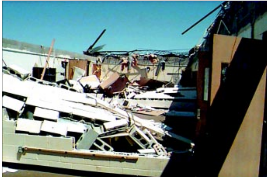
FIGURE 6-38: The non-reinforced interior CMU walls in this area of Kelly Elementary collapsed after the roof system was removed by vortex winds of a violent tornado.
