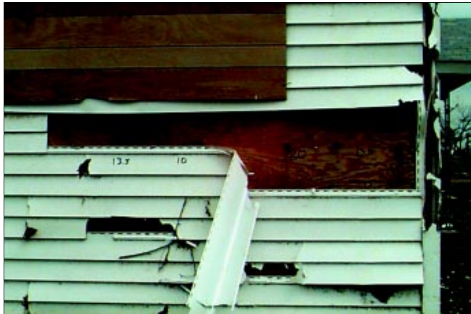
FIGURE 4-17: Some pieces of vinyl siding were blown off and in other areas the siding was torn away by missiles. The home was located along the periphery of a violent tornado in Mullhall, Oklahoma.
