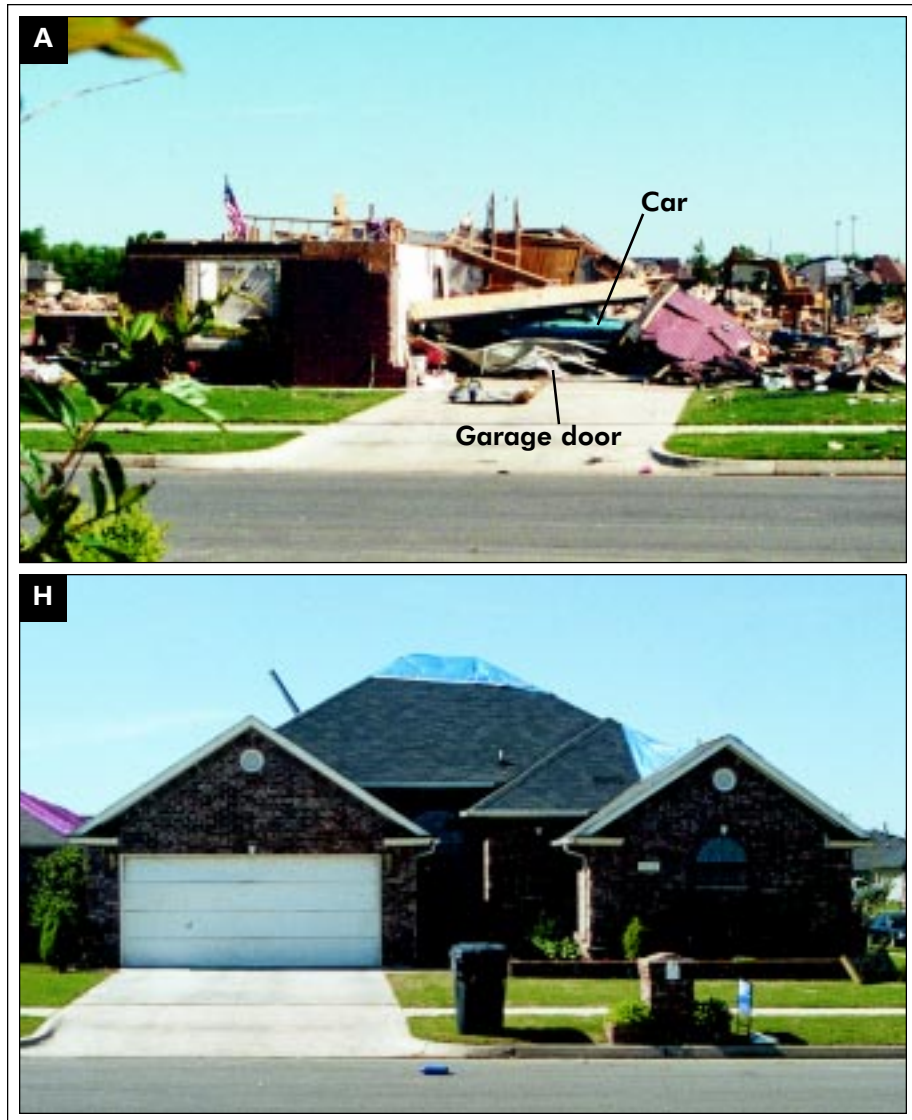
FIGURE 4-22: Home in Moore, Oklahoma, with partial roof loss and garage door in place (H) vs. home with total roof loss due to garage door failure (A) under positive pressure.
