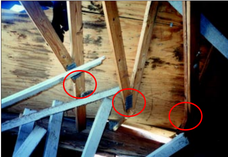
FIGURE 4-7: Roof truss failure. A single nail (circled) was used to connect each truss to the top plate. This house was in Midwest City, Oklahoma, and experienced inflow winds from a violent tornado.
