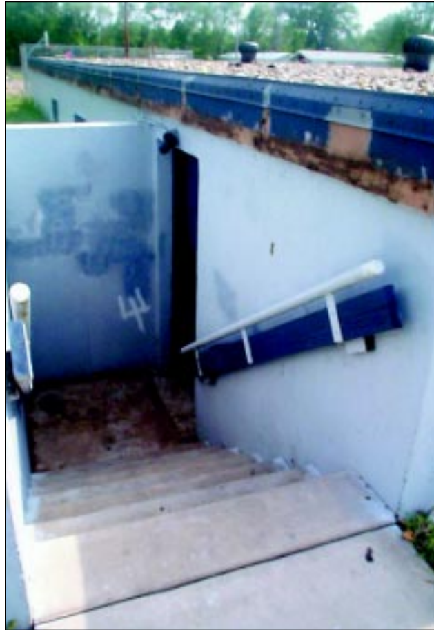
FIGURE 6-15: Stairway leading to entrance of manufactured home community shelter, Wichita, Kansas. The only means of accessing this structure were this stairway and an identical one at the other side of the shelter.
