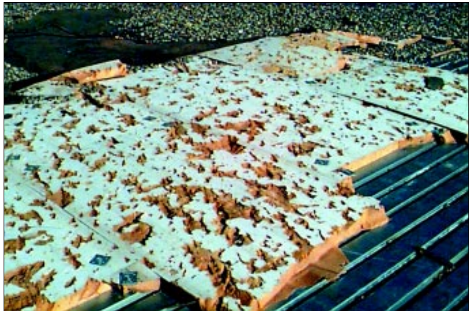
FIGURE 3-27: Close-up view of polyisocyanurate roof insulation boards (the boards are 4-ft by 8-ft) at Westmoore High School. This roof is approximately 25 feet above grade. Some of the missiles only caused superficial damage to the insulation; but several others had sufficient force to make large gouges in the insulation. For scale, the square metal fastener plates near the board corners are 3-in by 3-in.
