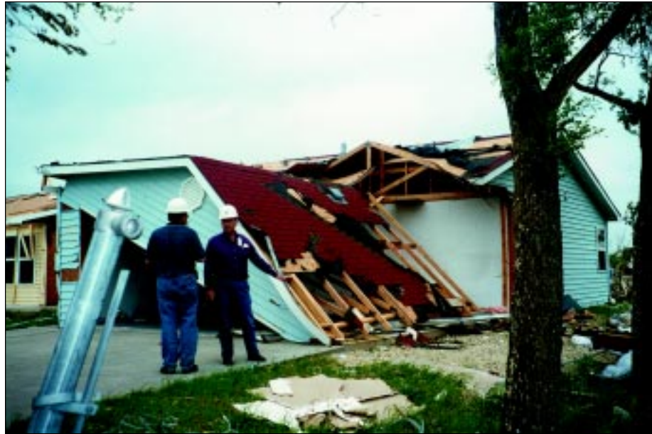
FIGURE 4-6: Wall failure due to inadequate lateral load resistance in Wichita, Kansas. The return wall at this garage was inadequate to carry wind loads and may have led to this failure.
