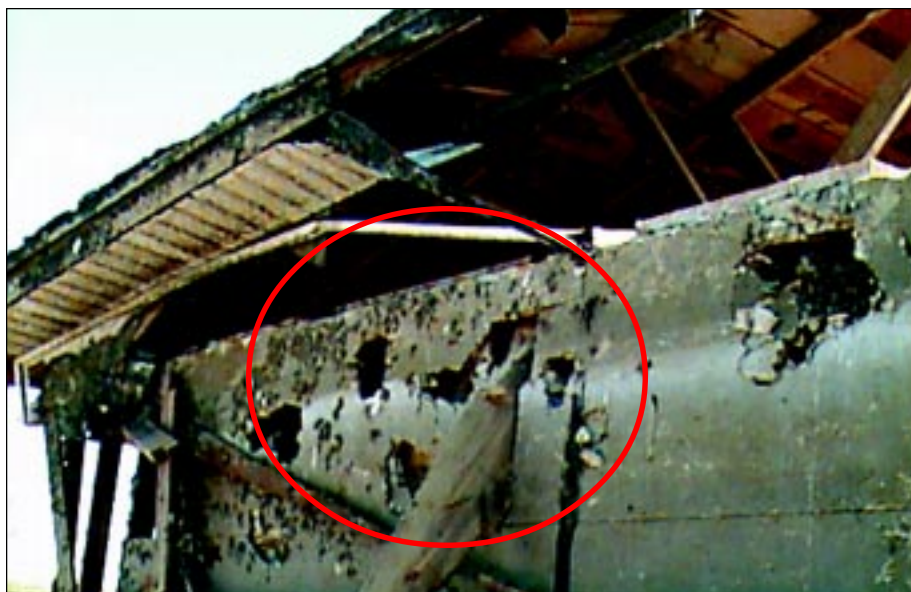
FIGURE 3-29: Several missiles struck the wall of this house in Del City, Oklahoma, including a medium sized piece of debris in the center of the photo.
