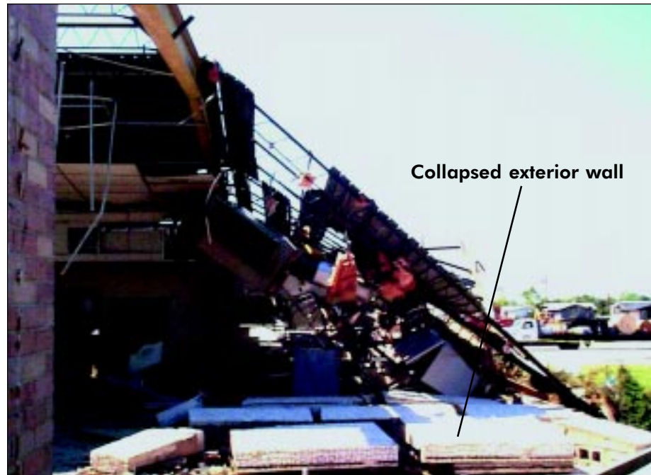
FIGURE 5-13: Collapsed roof structure and exterior wall at Kelly Elementary School in Moore, Oklahoma, struck by the vortex of a violent tornado.
