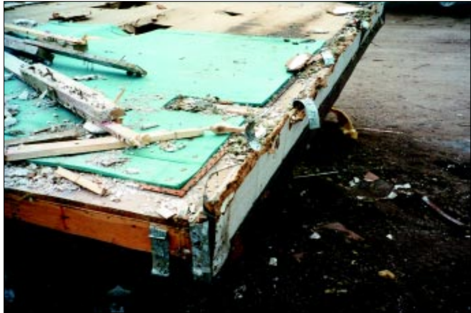
FIGURE 4-56: A close-up of the manufactured home floor and chassis after it was removed by a contractor from the permanent foundation in Figure 4-55.
