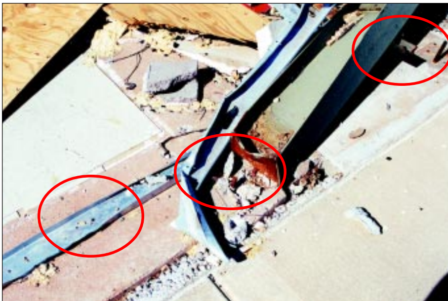
FIGURE 5-6: Attachment of columns to foundation and attachment of wall bottom plates to concrete slab. Regional outlet mall, Stroud, Oklahoma, hit by a strong tornado vortex.
