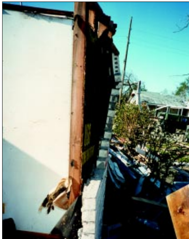
FIGURE 4-37: Failure of brick veneer wall, Del City, Oklahoma.
