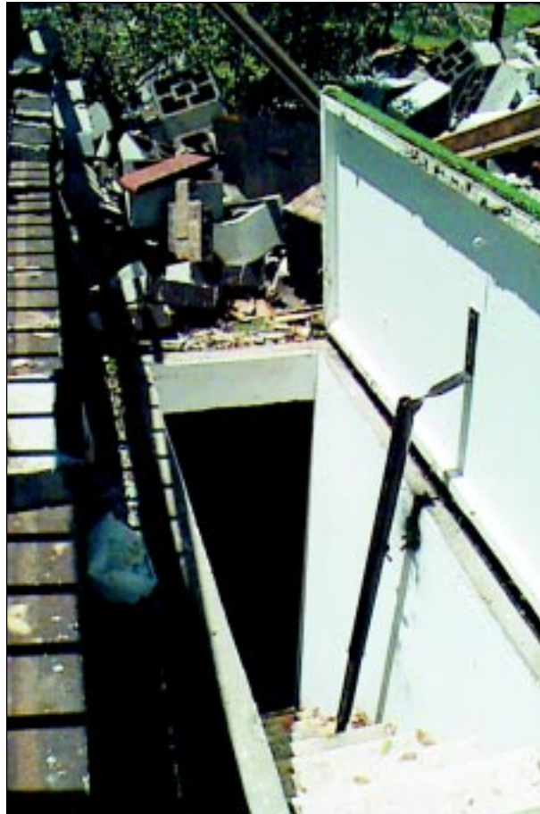
FIGURE 6-18: This belowground shelter is susceptible to water runoff.
