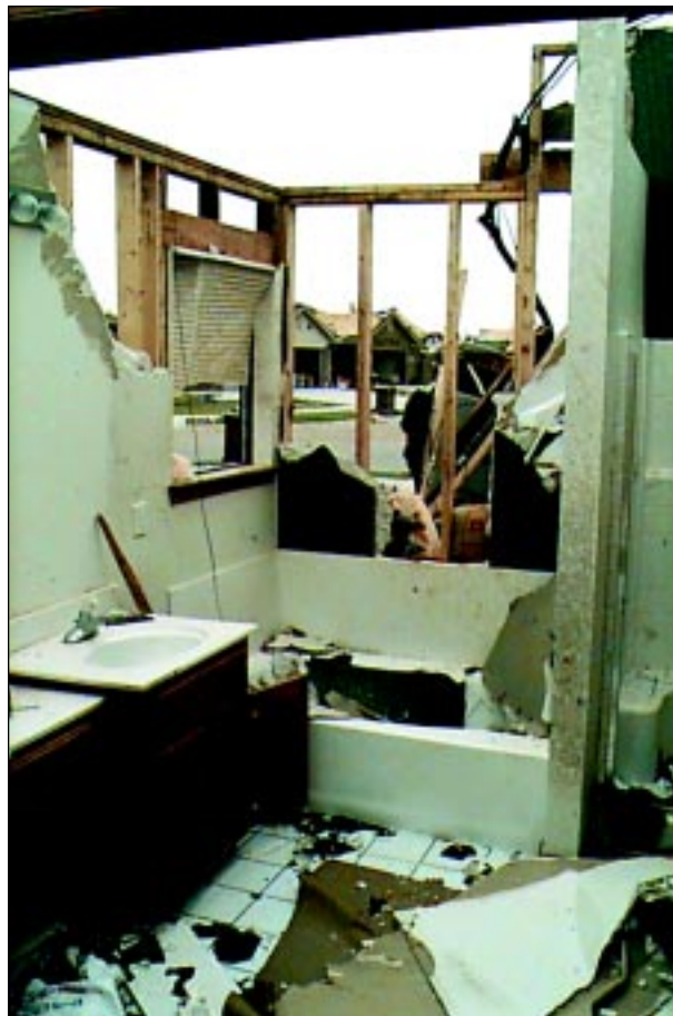
FIGURE 6-24: This bathroom was on an exterior wall and had a window. It did not provide a safe place of refuge.
