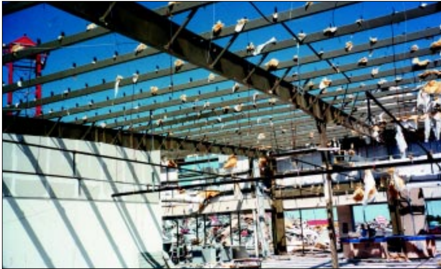
FIGURE 5-5: Metal roof deck (missing in photo) of regional outlet mall, Stroud, Oklahoma, was blown off when hit by a strong tornado vortex.
