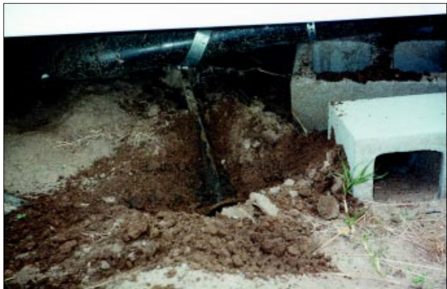
FIGURE 4-50: Ground anchor of manufactured home pulled from soil. This home in Wichita, Kansas, was located within the inflow area of a strong tornado.
