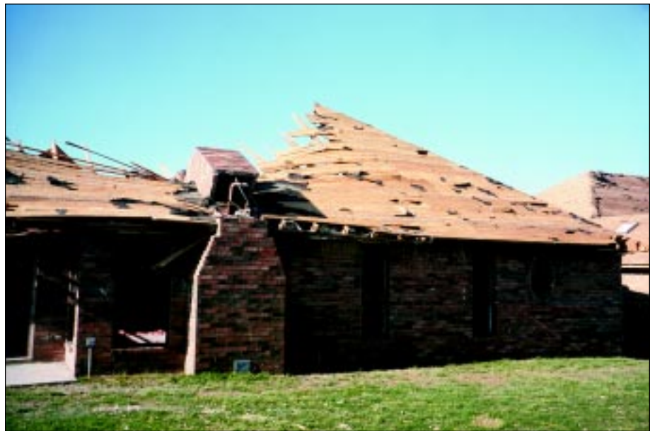
FIGURE 4-40: Failure of brick chimney onto roof of home located along the periphery of a violent tornado, Moore, Oklahoma.
