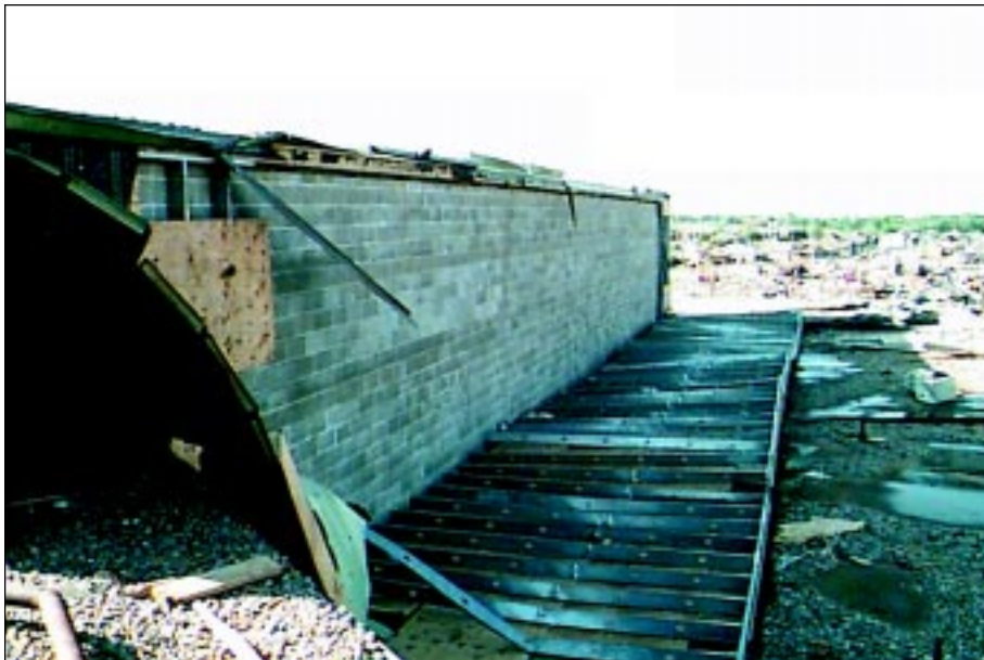
FIGURE 5-28: This metal-clad wall covering collapsed and in other areas it was blown completely away.
