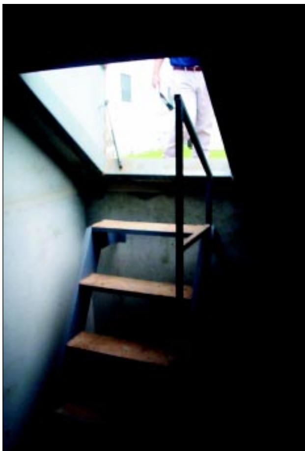
FIGURE 6-16: Stairway access to group shelter at manufactured home rental development, Wichita, Kansas, shown in Figure 6-9. This development was not affected by any of the tornadoes that struck on May 3, 1999.
