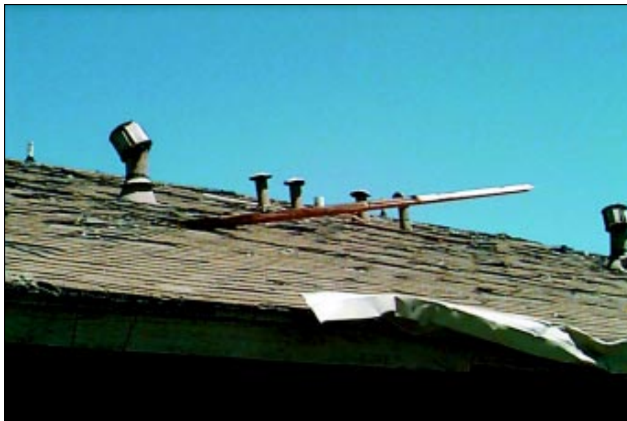
FIGURE 3-17: This missile struck a house located in Moore, Oklahoma.
