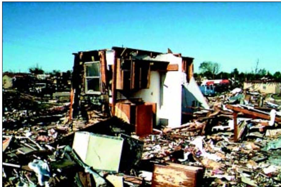
FIGURE 6-20: Interior core of house remains, consisting of a bathroom, closets, and a wall with kitchen cabinets after being struck by a strong tornado.
