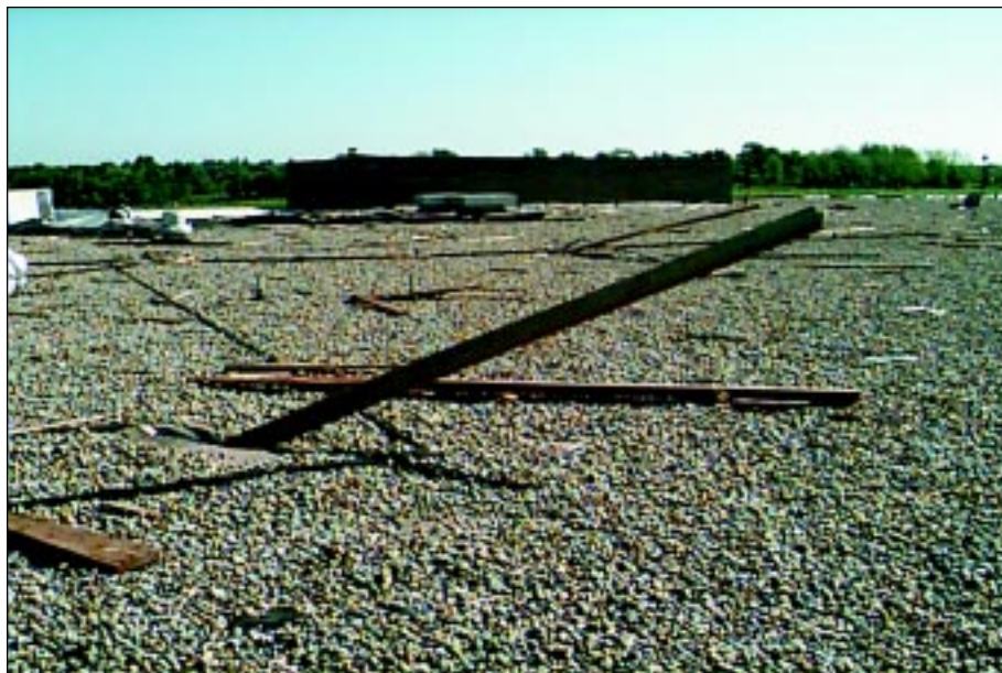
FIGURE 3-16: Medium and small missiles through and on Westmoore High School's roof, Moore, Oklahoma
