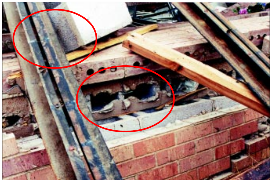
FIGURE 5-4: Failed structure showing broken deck welds (top circle), and no effective vertical reinforcement (bottom circle). Kelly Elementary School, Moore, Oklahoma, hit by vortex of violent tornado.
