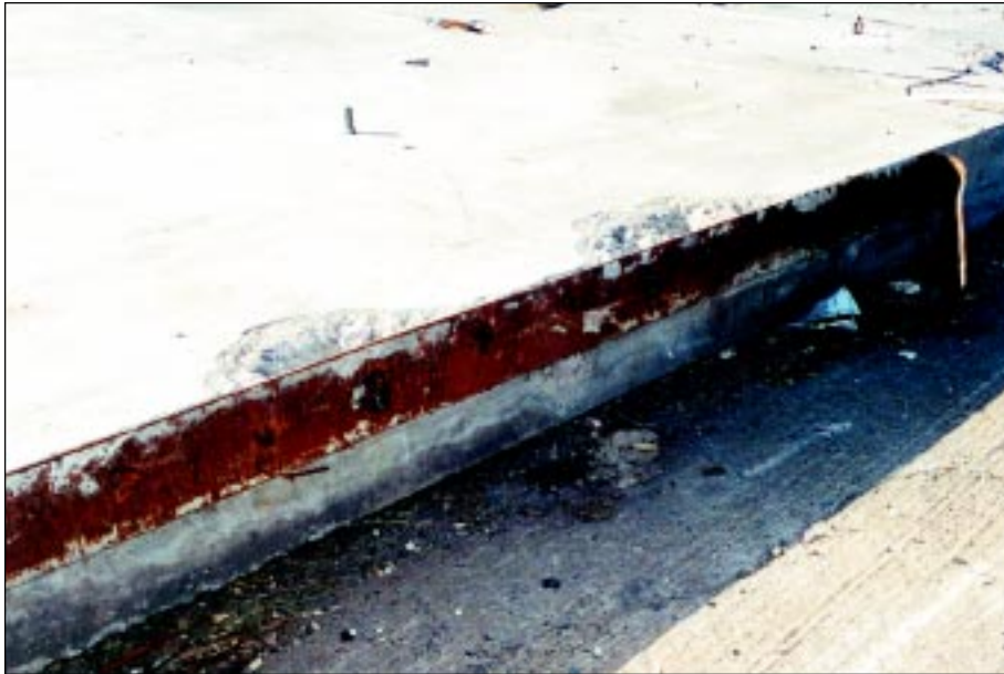
FIGURE 5-18: Top of failed tilt-up wall.
