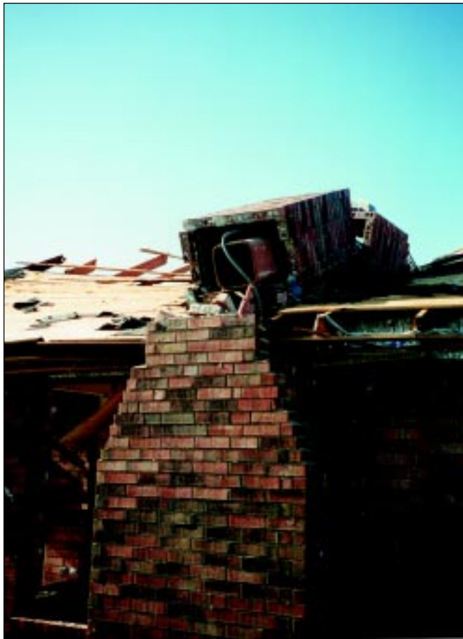
FIGURE 4-41: Close-up view of brick chimney failure in Figure 4-40.
