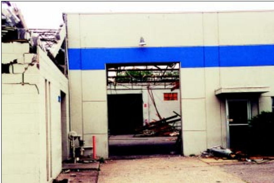
FIGURE 5-19: The tilt-up precast concrete walls in this building did not fail when the roof system failed. The masonry walls shown at the left of the photo were damaged. Note: many roof joists are still in place. Building was located in Wichita, Kansas, and was hit by weak tornado vortex.
