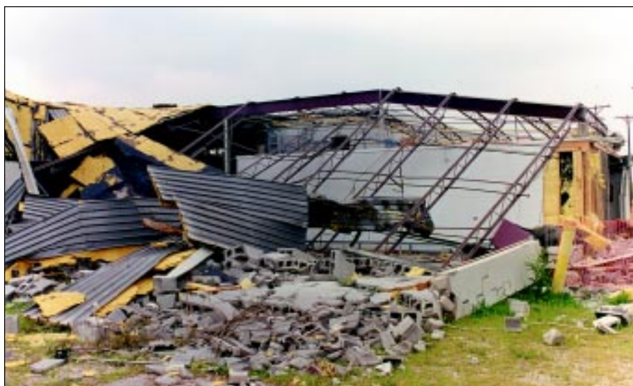
FIGURE 3-11: This un-reinforced masonry (URM) wall failed when inflow winds from a strong tornado acted on this building in Wichita, Kansas.
