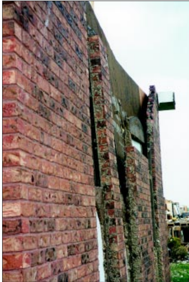
FIGURE 4-46: Failure of brick veneer in multi-family housing located along the periphery of a strong tornado, Wichita, Kansas.
