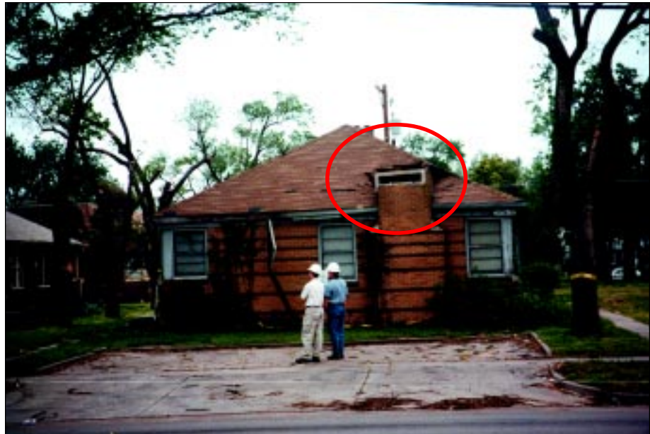
FIGURE 4-44: Chimney failure onto roof of single-family attached housing located along the periphery of a strong tornado, Wichita, Kansas.
