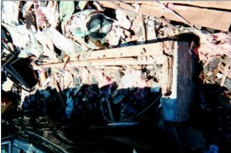
FIGURE 4-10: Wall framing to bottom plate failure. This house in Del City, Oklahoma, experienced a direct hit from the vortex of a violent tornado.
