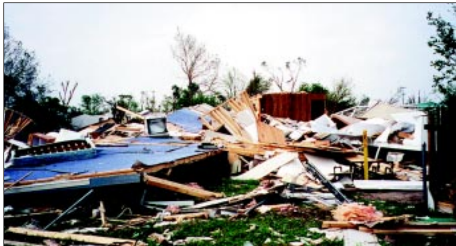
FIGURE 6-27: Damaged and destroyed manufactured homes on non-permanent foundations in Wichita, Kansas, that were in the direct path of a strong tornado.
