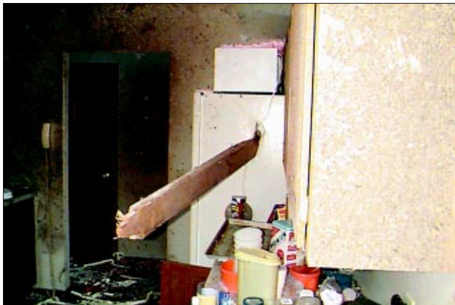
FIGURE 3-20: A 2-in by 6-in missile penetrating a refrigerator located inside a home in the Country Place subdivision outside Oklahoma City, Oklahoma.
