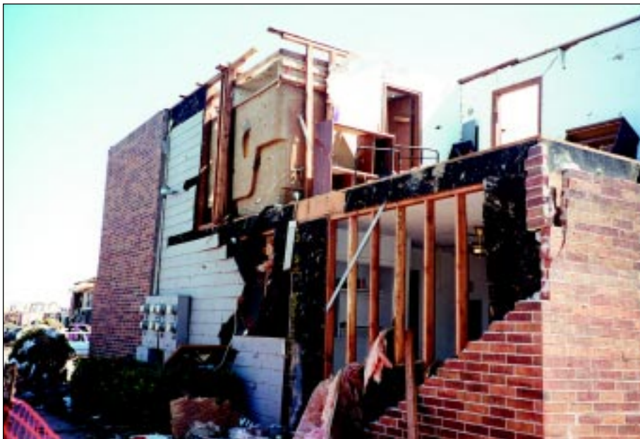
FIGURE 4-11: Stud-wall and sole-plate-to-floor failure on a second story wall. This multi-family residence in Moore, Oklahoma, was located a few hundred feet from the vortex of a violent tornado and was exposed to inflow winds.
