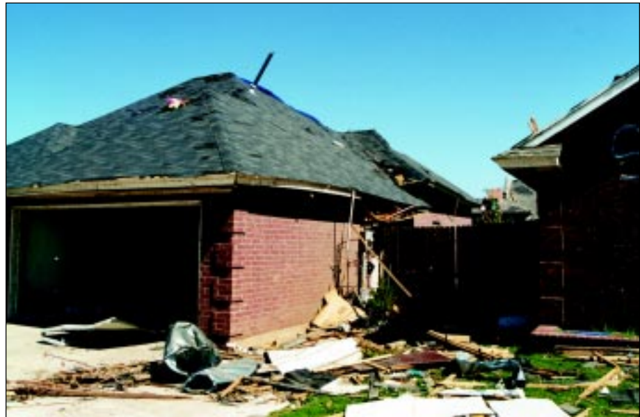
FIGURE 4-26: A 2x4 member extends out of the gap that runs the length of this garage wall between the top of the wall and the roof framing.
