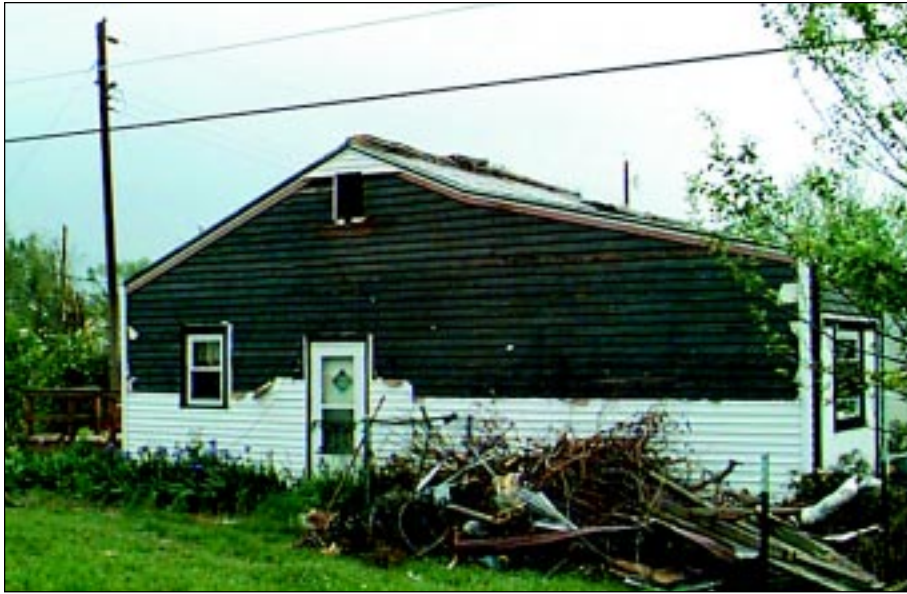
FIGURE 4-16: The vinyl (white) that was installed over wood siding experienced damage; however, the wood siding was undamaged. The home was located along the periphery of a violent tornado in Wichita, Kansas.
