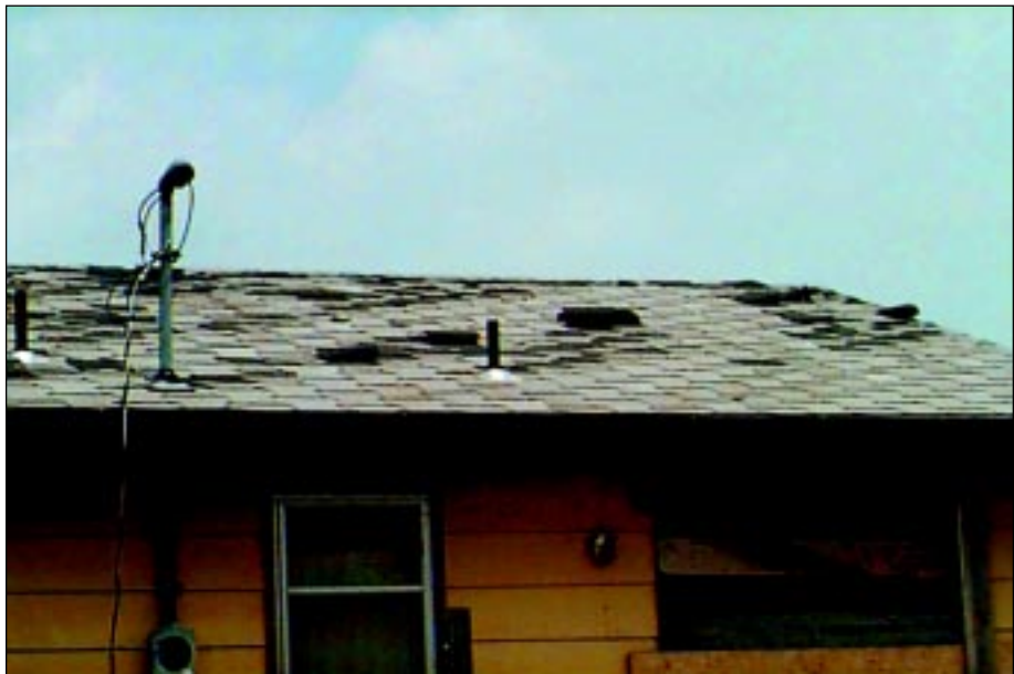
FIGURE 4-15: Several T-lock shingles on this house were lifted and torn. This house was on the periphery of a weak tornado in Wichita, Kansas.
