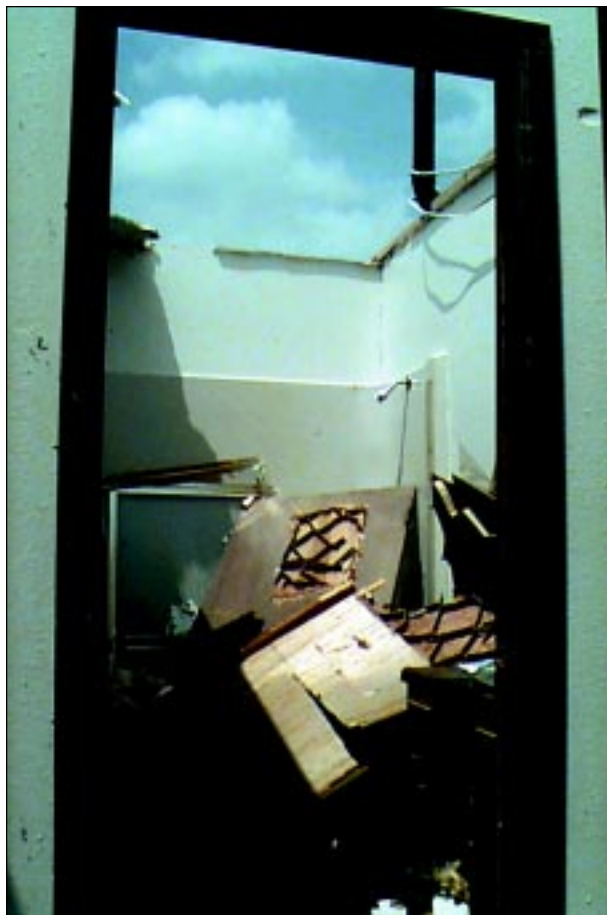
FIGURE 6-21: This apartment complex in Kansas was affected by inflow winds associated with a strong tornado. The roof and ceiling were blown off of the interior bathroom of this house, the door was blown into the bathroom, and the tub was full of debris. This bathroom would not have provided a safe place of refuge.
