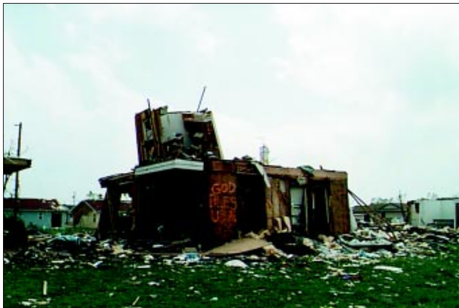
FIGURE 6-25: The second story of single-and multi-family houses typically experienced far greater damage than the first story. This multi-family home in Wichita, Kansas, was affected by inflow winds of a strong tornado.
