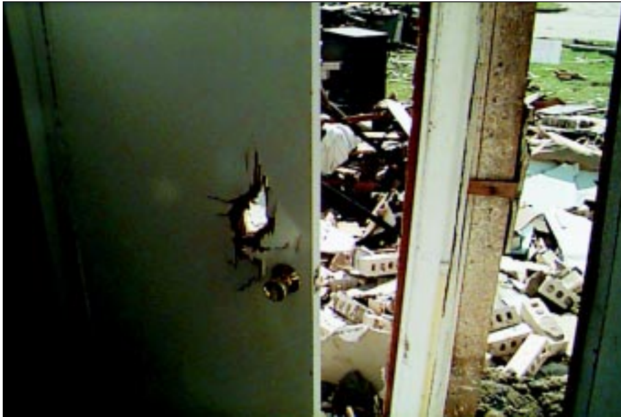
FIGURE 4-27: A missile penetrated this exterior door in Del City, Oklahoma. Interior hollow-core doors typically offer even less missile protection than common exterior doors.
