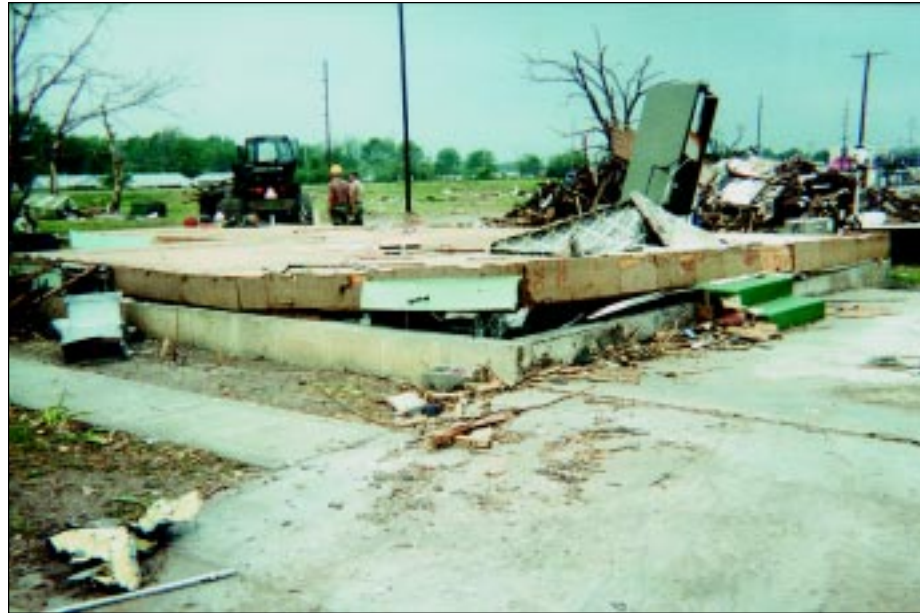
FIGURE 3-5: Wind uplift acting on this house in Haysville, Kansas, resulted in this corner of the building being lifted off its foundation.
