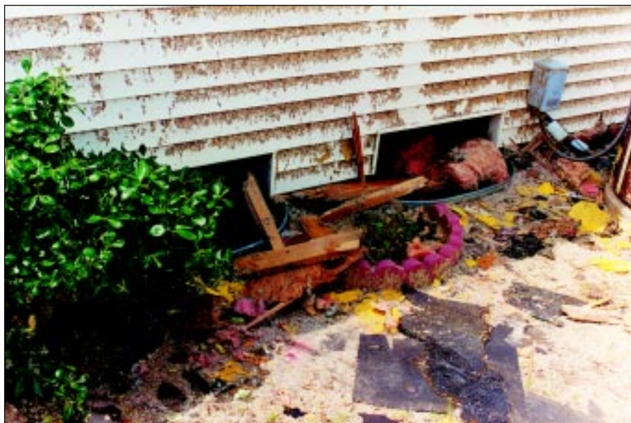
FIGURE 6-26: Basement windows of a single-family residence, showing vulnerability to debris.
