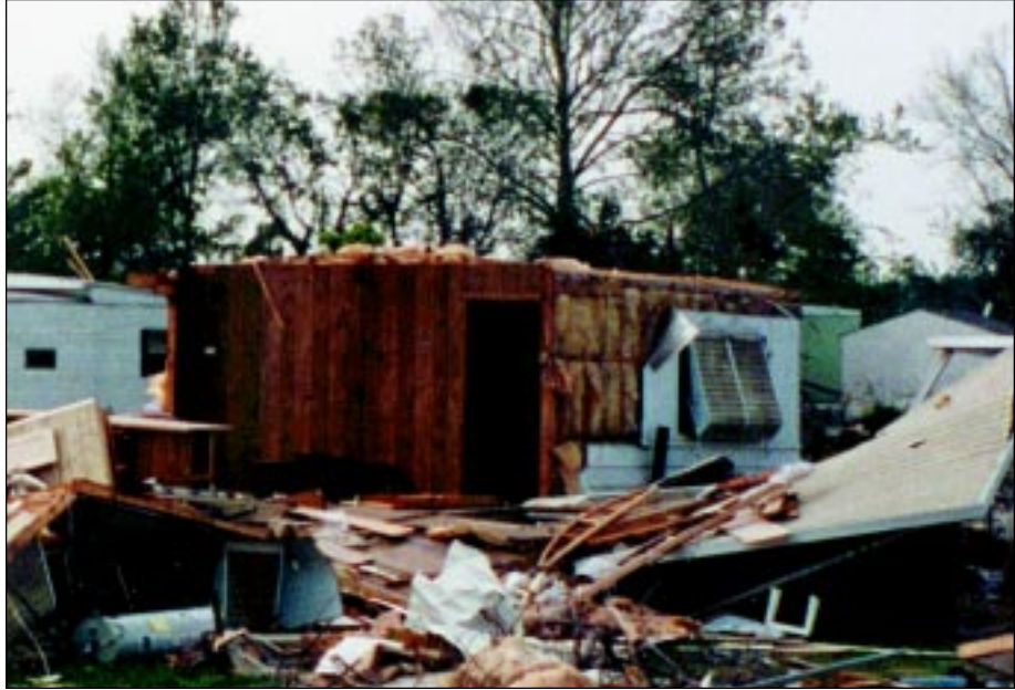
FIGURE 4-53: Manufactured home roof and wall damage experienced due to inadequate resistance to lateral and uplift wind forces associated with straight inflow winds of a weak tornado, Wichita, Kansas.
