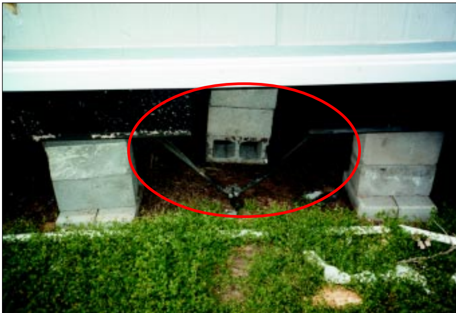
FIGURE 4-59: View of anchor strap and attachment indicating some lateral shifting of a manufactured home located along the periphery of a violent tornado, Wichita, Kansas.
