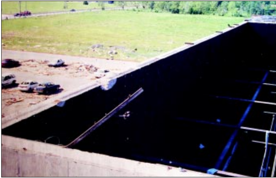
FIGURE 5-14: Roof blown off over top of auditorium at Westmoore High School, Moore, Oklahoma, hit by inflow winds of violent tornado.
