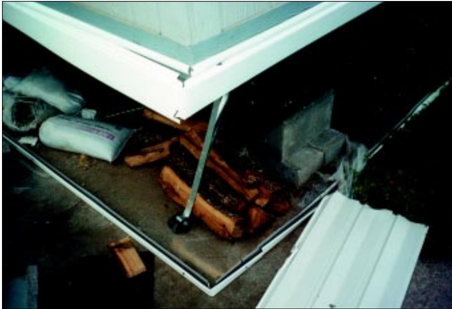
FIGURE 4-58: View of anchor strap and attachment indicating lateral shifting of a manufactured home, Haysville, Kansas. This home was located along the periphery of a violent tornado.
