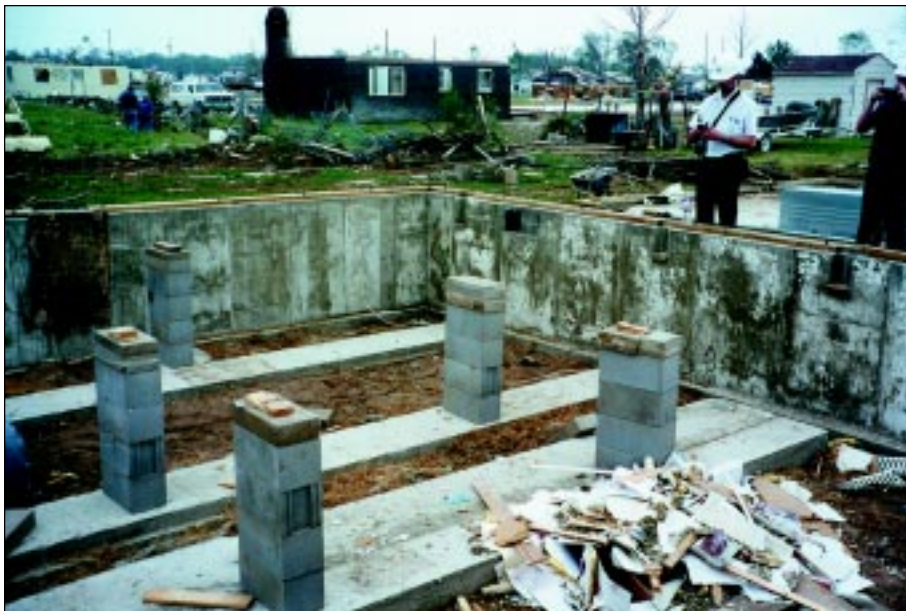
FIGURE 4-55: Lack of bolts or positive connectors present between the chassis and foundation of a double-wide manufactured house, Haysville, Kansas. The floor framing of the house was still resting on the foundation after the tornado passed.
