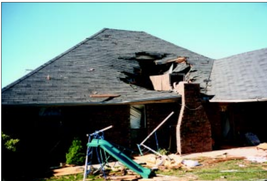
FIGURE 4-42: Failure of brick chimney onto top of home located along the periphery of a violent tornado, Moore, Oklahoma.
