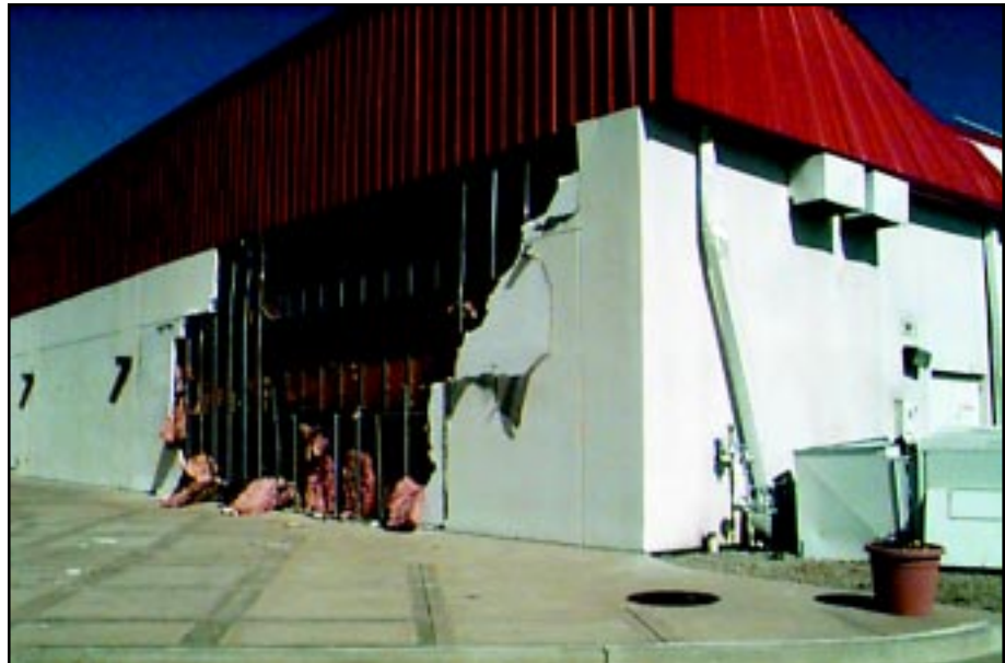
FIGURE 3-10: EIFS and metal fascia damage at the regional outlet mall in Stroud, Oklahoma. This is a typical example of a components and cladding failure.
