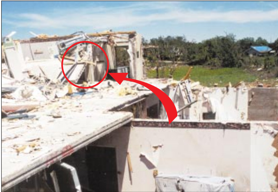
FIGURE 5-21: Hollow-core plank formed on second floor of a Midwest City, Oklahoma, hotel that was struck by the vortex of a strong tornado.
