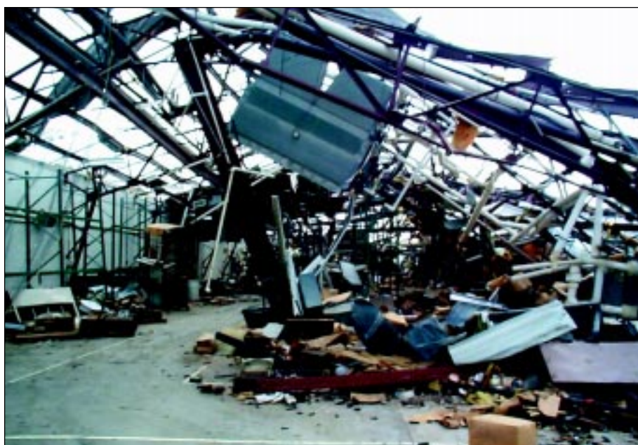
FIGURE 3-12: The vortex of a violent tornado passed within 100 yards of this plastics manufacturing plant in the city of Haysville, Kansas. The wind forces caused the failure of its primary structural system: a pre-engineered steel frame with masonry infill walls.
