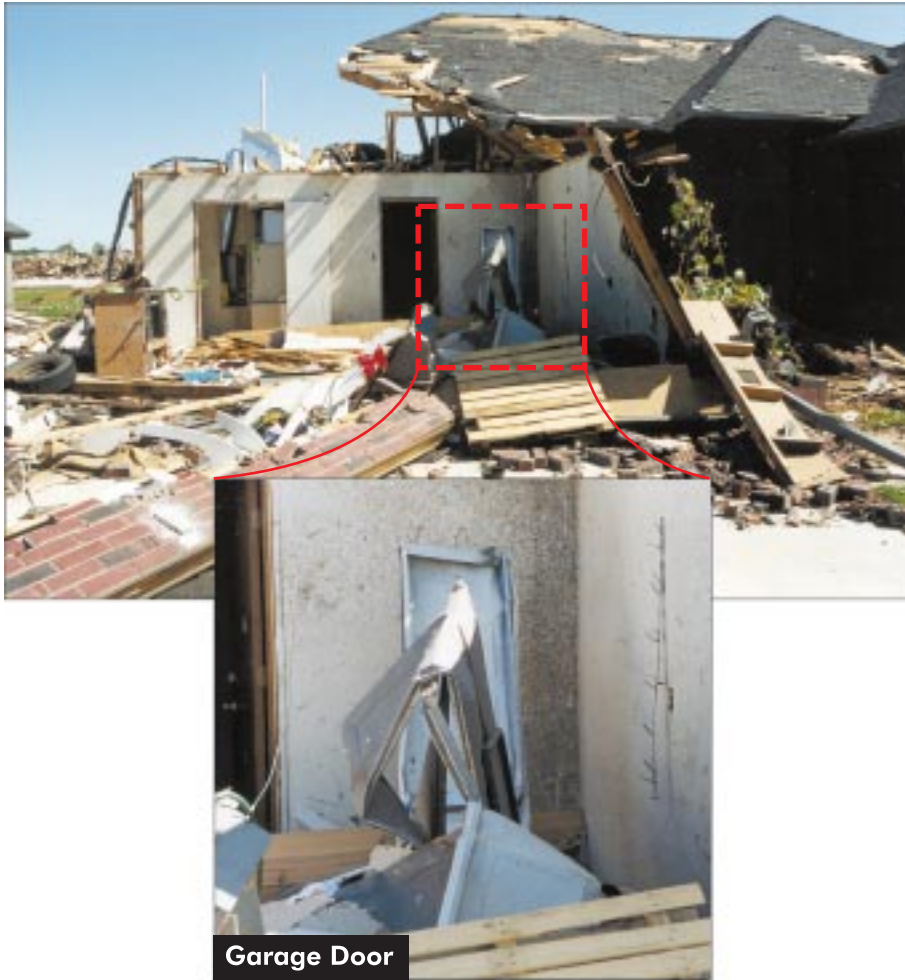
FIGURE 4-23: Garage door failure possibly resulting in the localized partial roof failure on the left side of this home located in Moore, Oklahoma.
