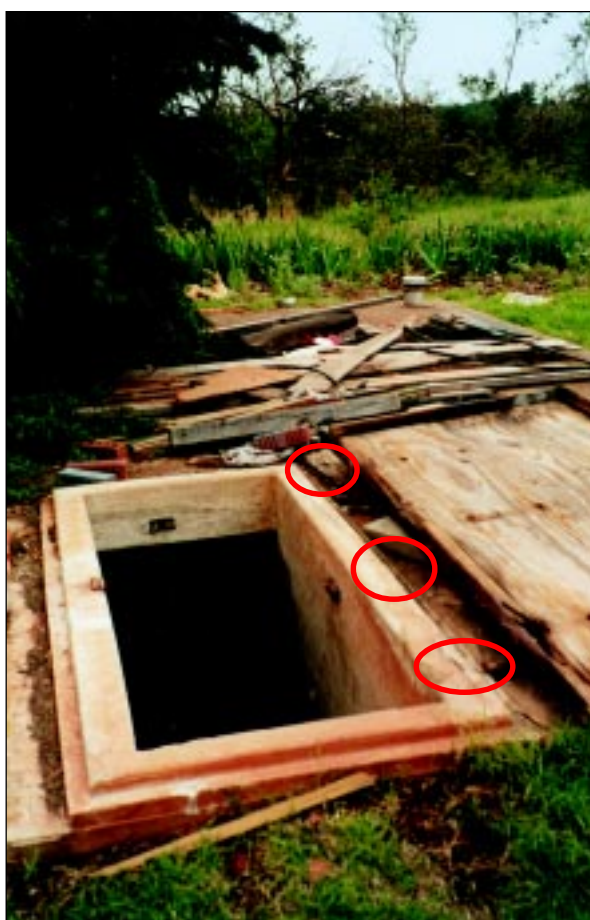
FIGURE 6-11: Door to underground shelter with rotting wood and corroded hinges.
