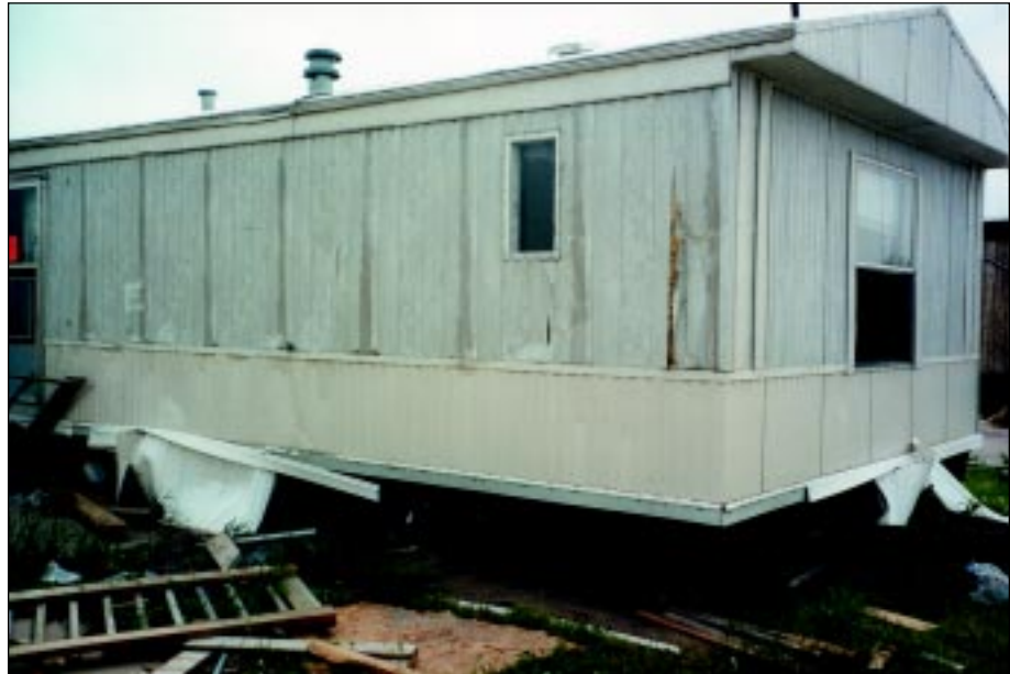
FIGURE 4-57: This manufactured home laterally shifted from wind force generated along the periphery of a violent tornado, Haysville, Kansas.
