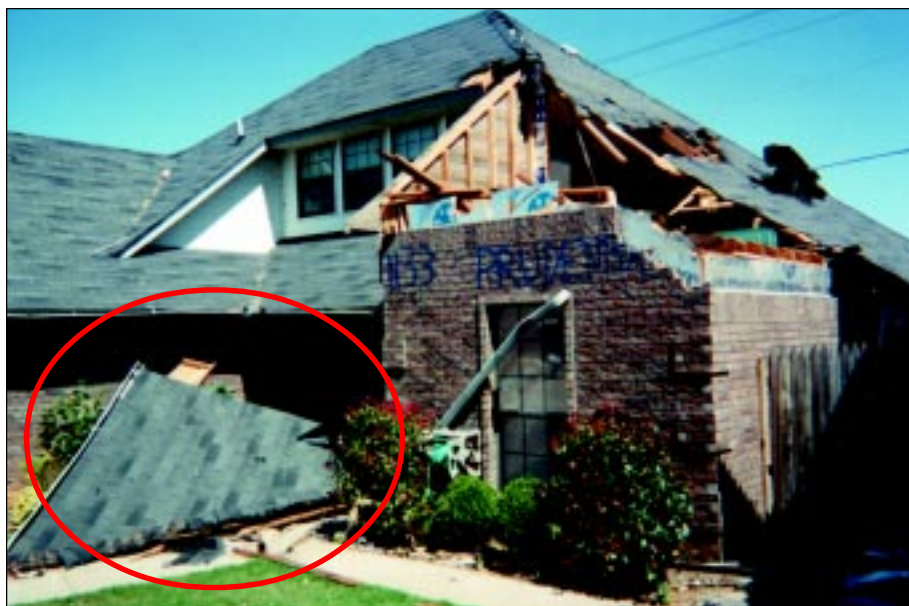
FIGURE 3-7: Failure of hip roof due to internal pressures and leeward roof (uplift) wind forces acting together. This house, which was exposed to inflow winds on the periphery of a violent tornado, is located in a suburb of Oklahoma City, Oklahoma.
