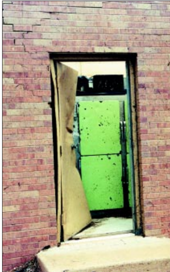
FIGURE 5-32: Damaged door most likely opened by impact with heavy object. Kelly Elementary School, Moore, Oklahoma.
