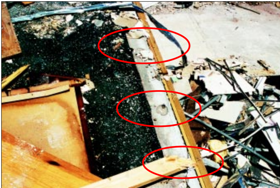
FIGURE 5-22: Attachments of lower plates for wall to hollow core plank using powder driven anchors failed when required to carry loads generated by the winds of a strong tornado vortex. This motel was located in Midwest City, Oklahoma.
