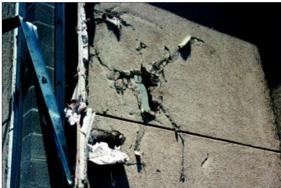
FIGURE 6-37: This EIFS wall system was penetrated by numerous windborne missiles.
