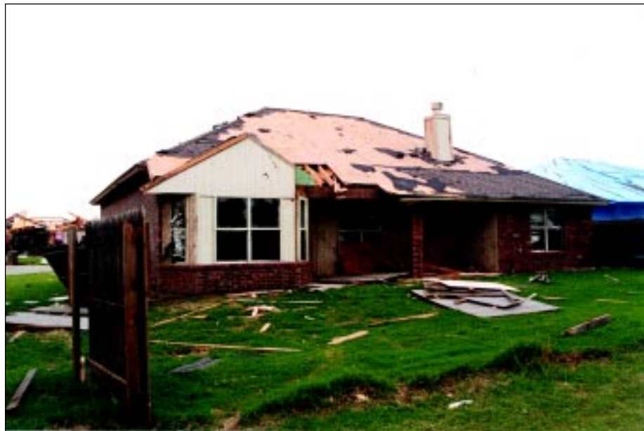
FIGURE 4-28: Damage to back of home in the Country Place Subdivision in Oklahoma City, was limited to several window failures and roof covering damage. The home was located along the periphery of a violent tornado.
