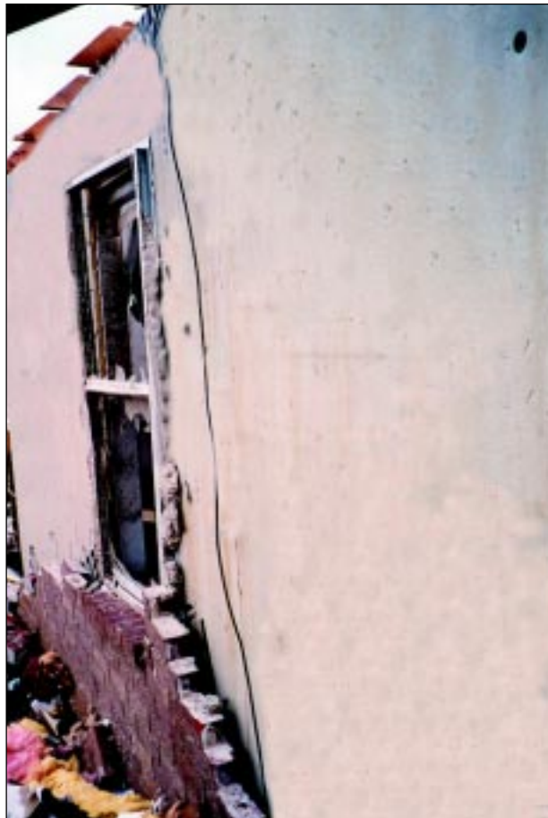
FIGURE 4-35: Inadequate bonding of mortar to galvanized brick ties contributed to this masonry failure at a home in Bridge Creek, Oklahoma.
