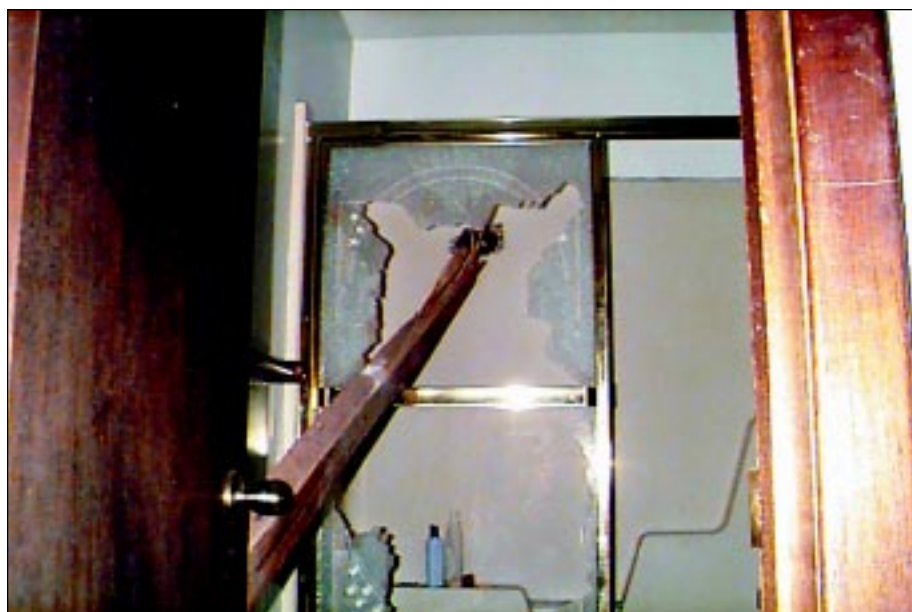
FIGURE 6-22: A 10-ft long 2-in by 6-in missile penetrated the exterior wall of an apartment in this multi-family house, which was sheathed with hardboard panels. The missile, which was generated from the vortex of a strong tornado, then penetrated the gypsum board and plastic tile tub enclosure, the tempered glass shower door, and the interior partition near the door frame. At the interior partition, it pierced through a stud and projected a few inches into the hallway (Figure 6-23).
