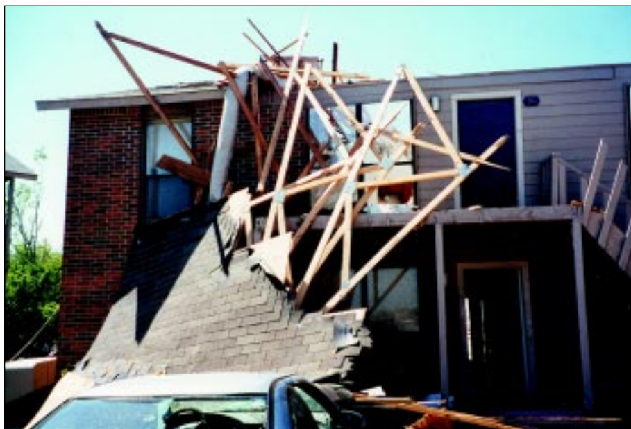
FIGURE 3-15: These trusses and roof covering (still attached to the roof sheathing) were displaced by the winds of a violent tornado and are capable of becoming large, windborne missiles. These trusses were originally attached to this apartment building.
