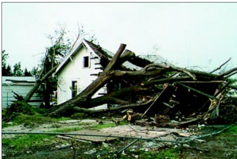
FIGURE 3-24: This building was on the periphery of a violent tornado damage area in Haysville, Kansas. One large tree fell near the corner of the house and collapsed a large portion of the roof and the corner walls. A smaller tree caused minor damage on the other corner of the house.
