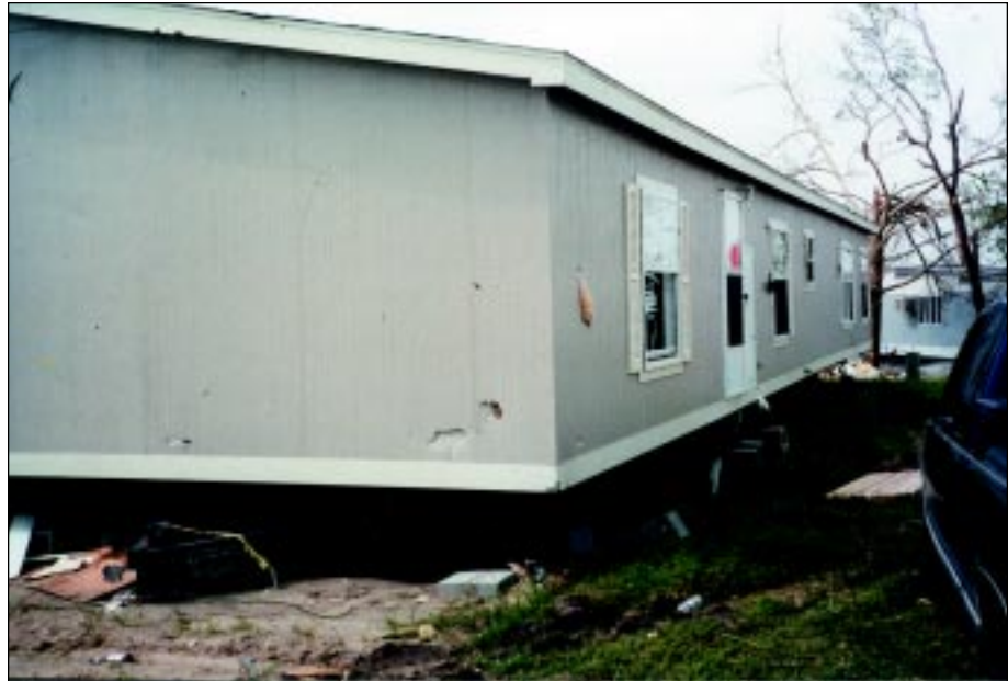
FIGURE 4-60: Manufactured home laterally shifted off its dry-stacked masonry block foundation from wind force generated along the periphery of a violent tornado, Wichita, Kansas.
