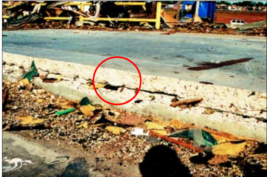
FIGURE 5-16: Failure of tilt-up concrete wall in Del City, Oklahoma, hit by inflow winds of a violent tornado.
