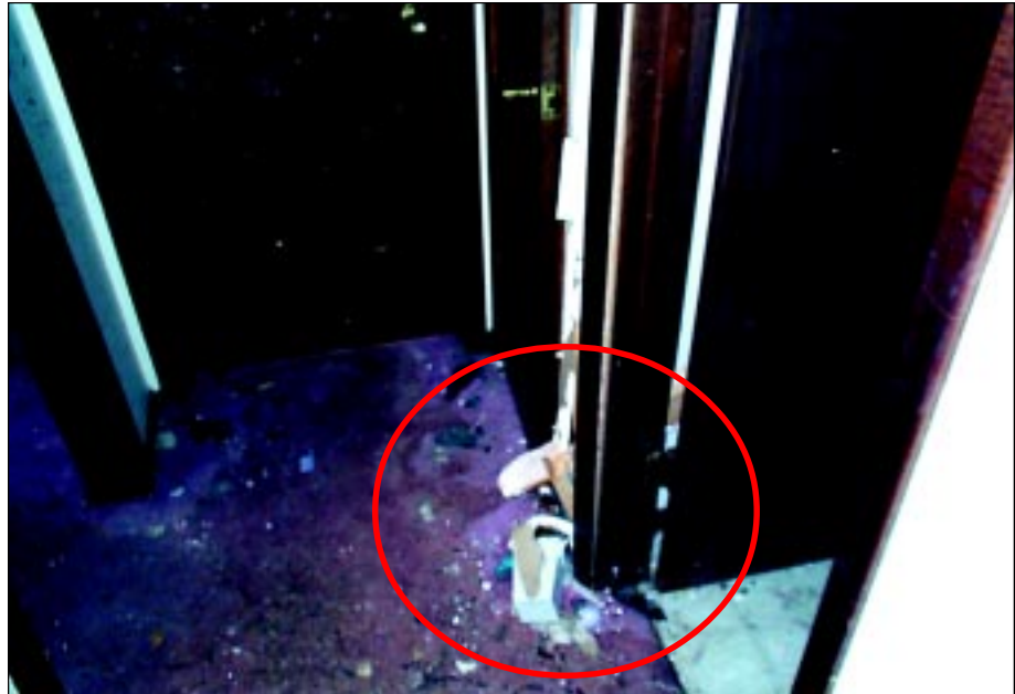
FIGURE 6-23: The missile in Figure 6-22 impacted and broke a 2-in by 4-in stud after traveling through the bathroom.
