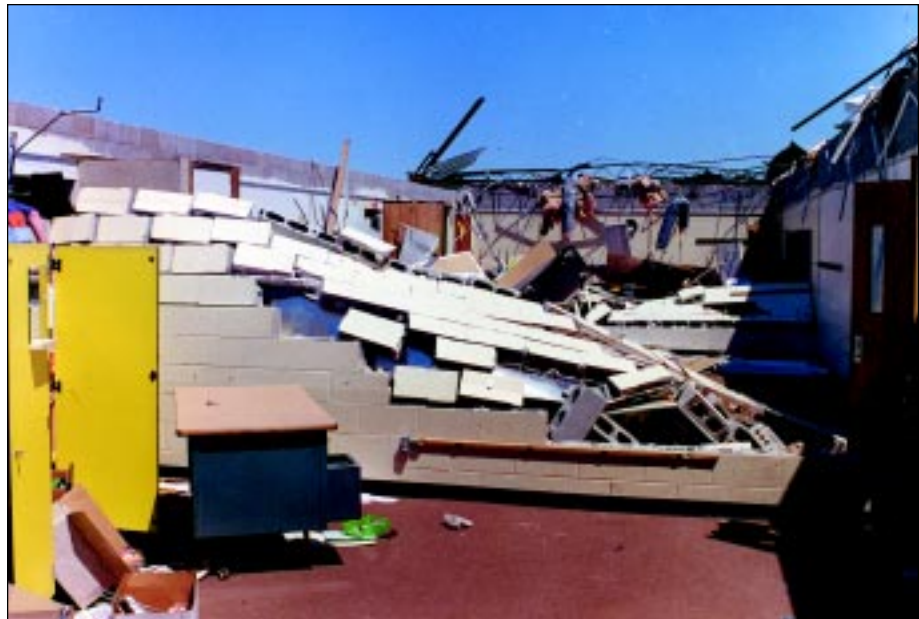
Figure 5-20: Damage to interior and exterior unreinforced masonry walls when bond beams failed at Kelly Elementary School in Moore, Oklahoma. The school was struck by the vortex of a violent tornado.
