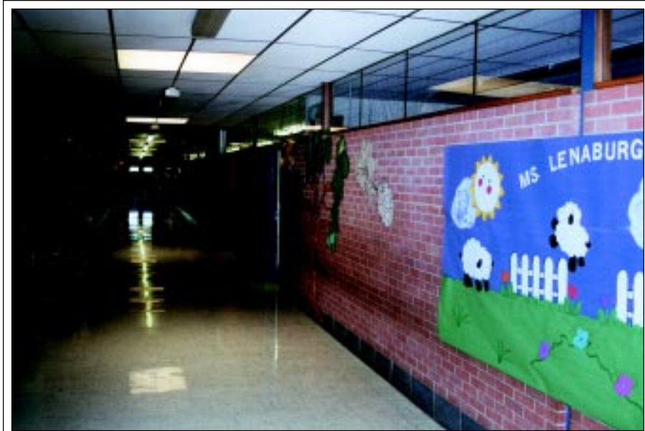
FIGURE 6-34: Northmoor Elementary place of refuge, Moore, Oklahoma – corridor with clerestory windows. This corridor offers little protection from tornadoes as shown in a school of similar design in Figure 6-35.
