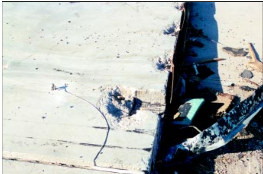
FIGURE 5-17: Top of failed tilt-up end wall.
