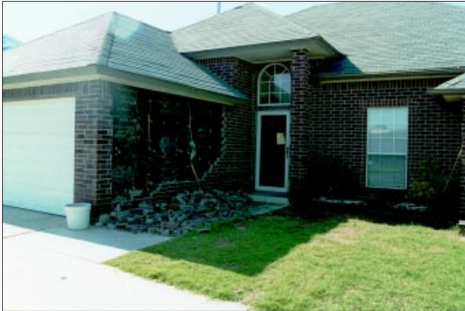
FIGURE 4-38: Failure of brick veneer wall, collapsed on the ground. This home, located outside Oklahoma City was on the periphery of a violent tornado.
