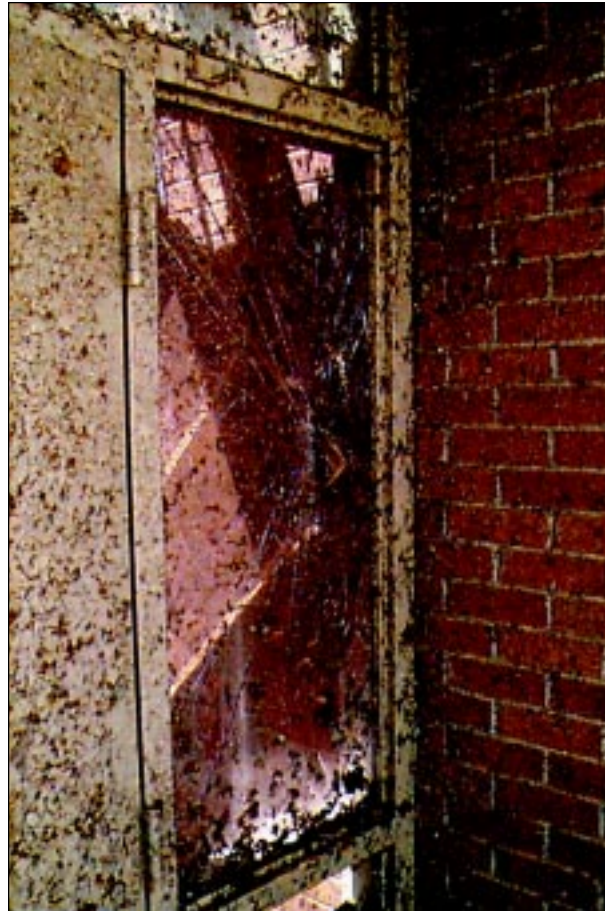
FIGURE 5-29: The corner of a table penetrated this laminated glass, but the glass remained in its frame. This school suffered major damage from inflow winds of a violent tornado in Moore, Oklahoma.
