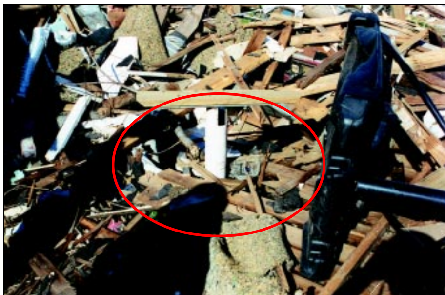
FIGURE 6-17: Heavy gauge ventilation pipe for a belowground shelter in Oklahoma withstood considerable debris impact.
