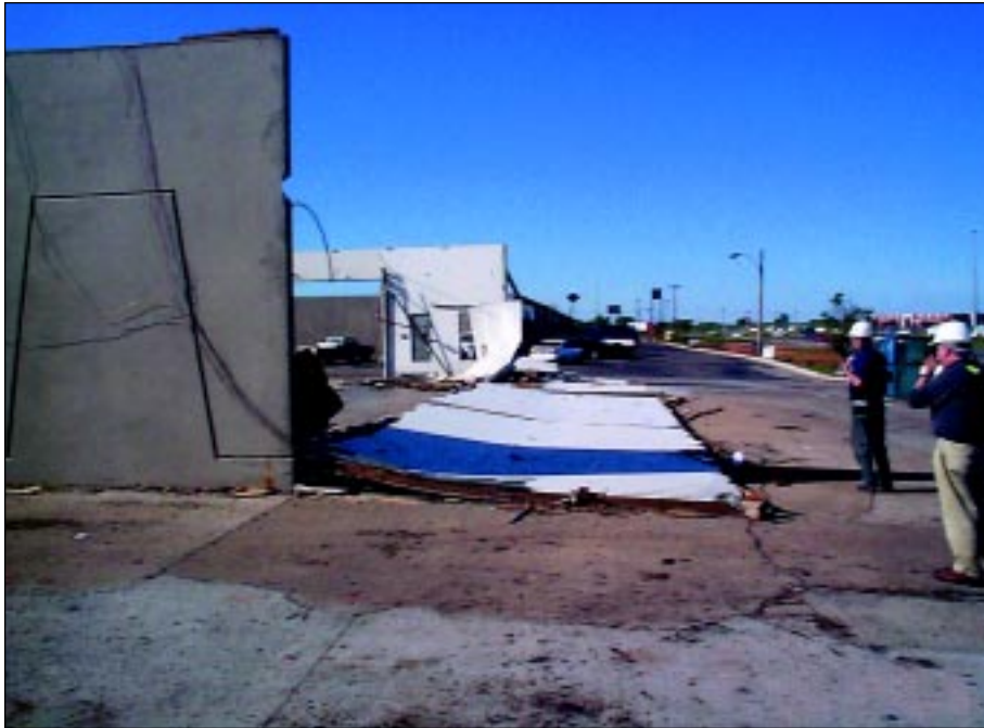
FIGURE 5-2: Tilt-up precast concrete walls at a storage building located outside Del City, Oklahoma. After the roof joists separated from the walls, this end wall became unable to withstand suction forces and failed.
