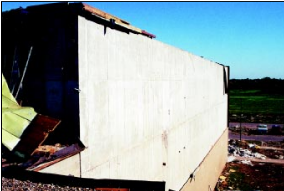
FIGURE 5-15: Exterior view of an undamaged reinforced concrete wall, Westmoore High School, Moore, Oklahoma, hit by inflow winds of a violent tornado. Note: decorative metal wall covering was peeled from this wall.
