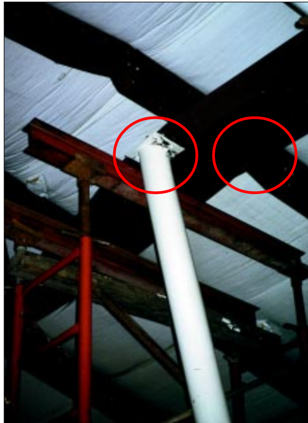
FIGURE 5-12: Out-of-plane buckling of the main girder supporting the roof created by a combination of uplift and horizontal wind loads. Plastics plant, Haysville, Kansas, hit by violent tornado. This building was in the inflow area of a strong tornado.
