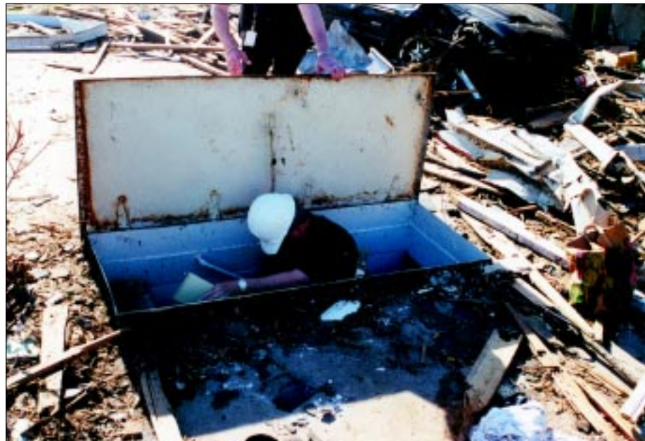
FIGURE 6-5: Del City storm cellar constructed of welded steel sheets with a concrete roof slab. This area was directly struck by the vortex of a violent tornado.
