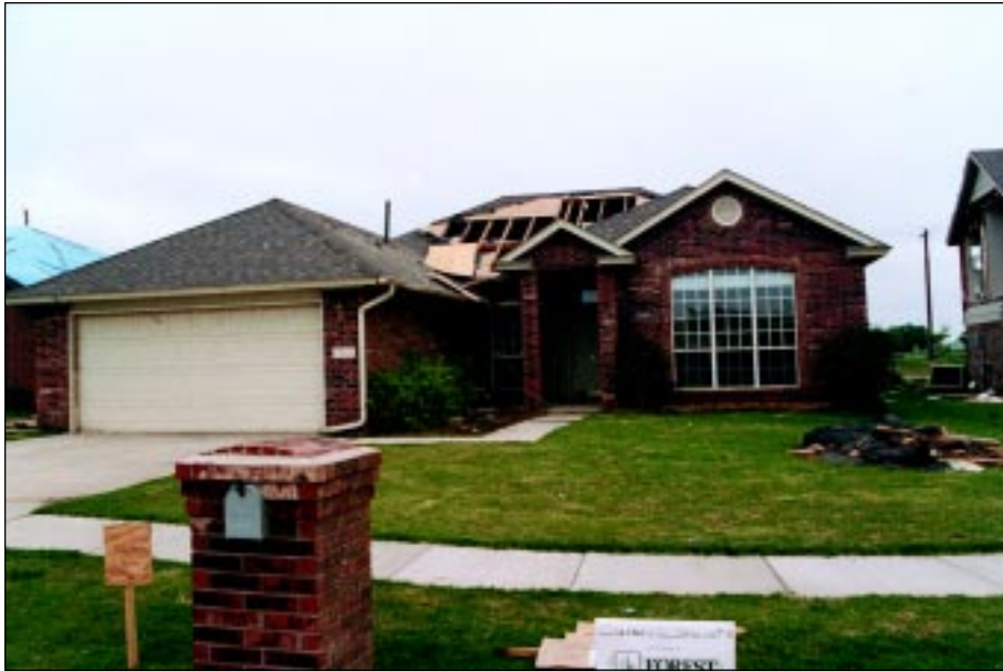
FIGURE 4-29: Front of home in Figure 4-28 where several pieces of roof sheathing failed.
