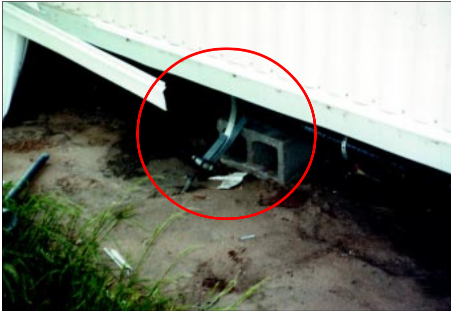
FIGURE 4-51: Anchor of manufactured home bent and pulled up from soil. This home in Wichita, Kansas, was located within the inflow area of a strong tornado.
