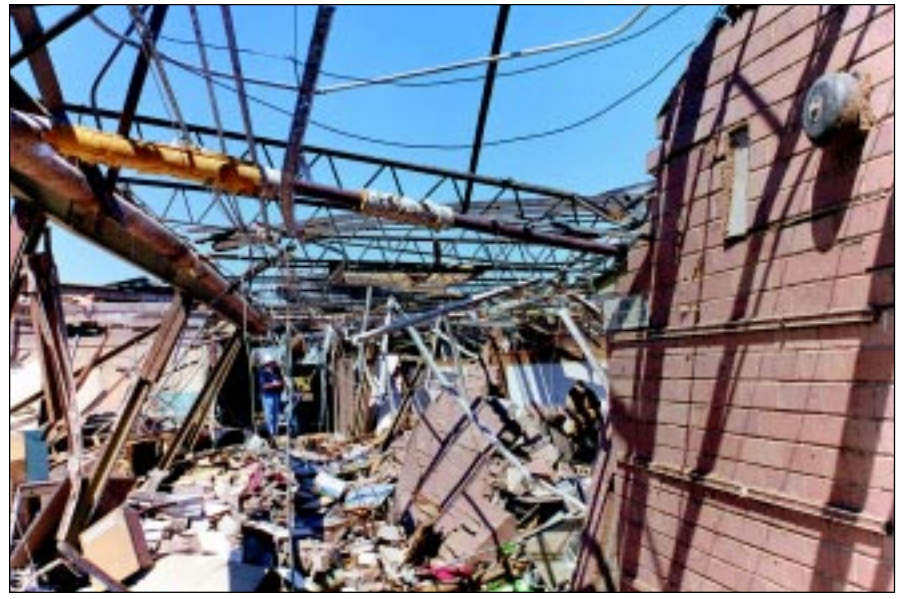
FIGURE 6-35: Kelly Elementary School, Moore, Oklahoma, place of refuge – corridor with clerestory windows. These interior corridor walls had brick masonry up to a height of approximately 7 ft. Glass extended from the top of the brick masonry to the top of the wall.
