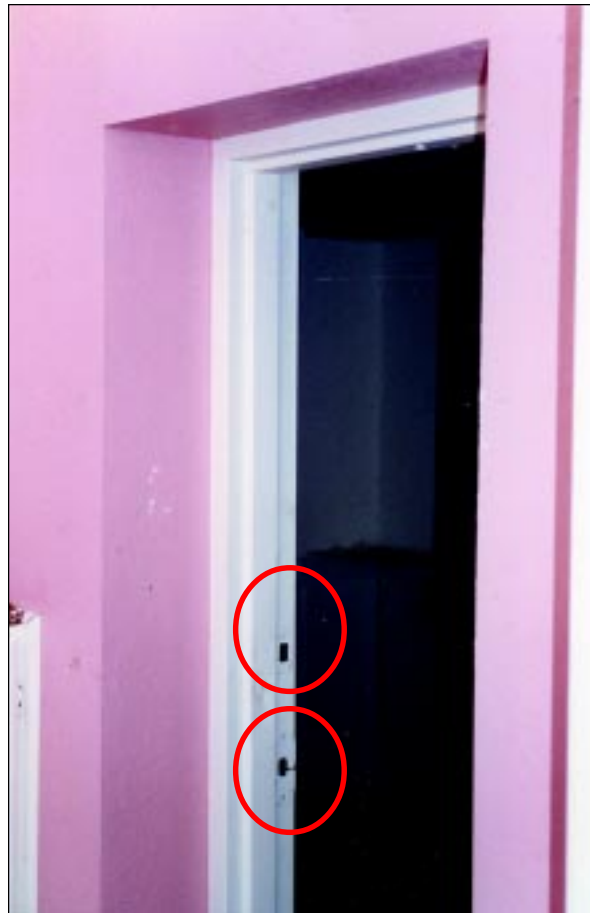
FIGURE 6-13: Shelter door of home in Del City, Oklahoma, showing an insufficient deadbolt locking device. The bottom circled area on the door frame is the catch for the only latching mechanism on the door. Note: the second opening in the door frame was not used to provide a second latching point (top circled area).
