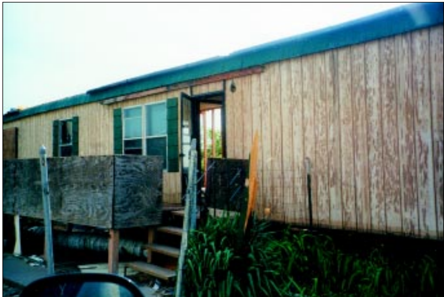
FIGURE 4-54: Damage to a manufactured home located on the periphery of a strong tornado, Wichita, Kansas.
