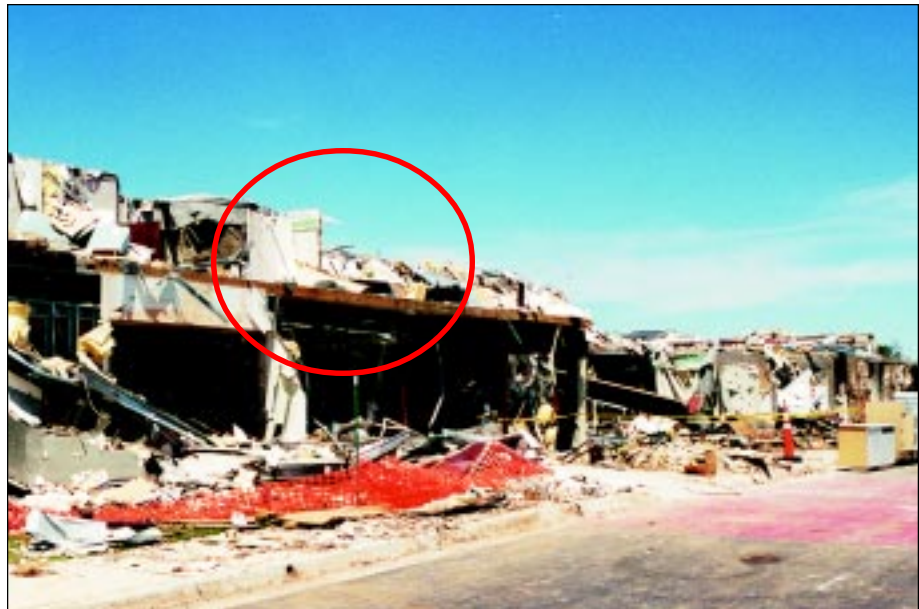
FIGURE 5-11: Motel in Midwest City, Oklahoma that experienced major damage when struck by the vortex of a violent tornado.
