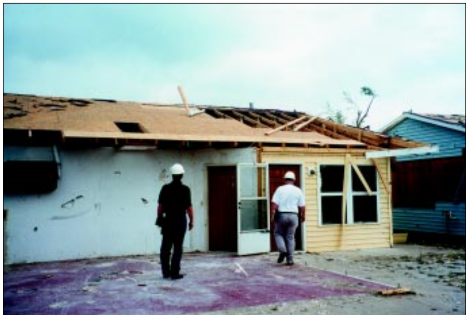
FIGURE 4-4: Although roof sheathing was lost at this Wichita, Kansas, home, code requirements of staggering joints in sheathing applications was observed. This house experienced inflow winds from a strong tornado.
