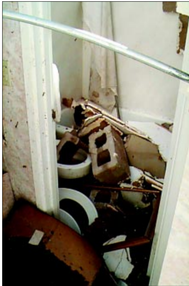
FIGURE 6-39: The roof and ceiling over this interior bathroom blew off. CMU from a firewall a few feet away blew into the bathroom, which was located on a motel's second floor in Midwest City, Oklahoma. This bathroom would not have provided a safe refuge.
