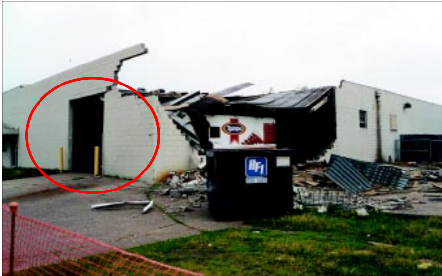
FIGURE 5-30: Failure of roof and walls on structure due to increased loads caused by initial failure of a rollup door, Wichita, Kansas.
