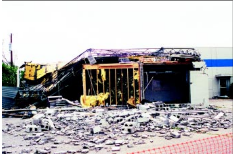
FIGURE 5-31: Additional structural damage caused by breach of envelope in Wichita, Kansas.
