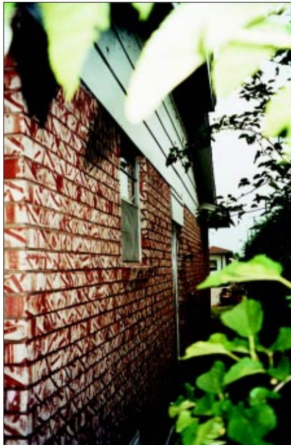
FIGURE 4-31: This brick veneer appears to be undamaged but close inspection indicated that this wall could be deflected inward with only hand pressure.
