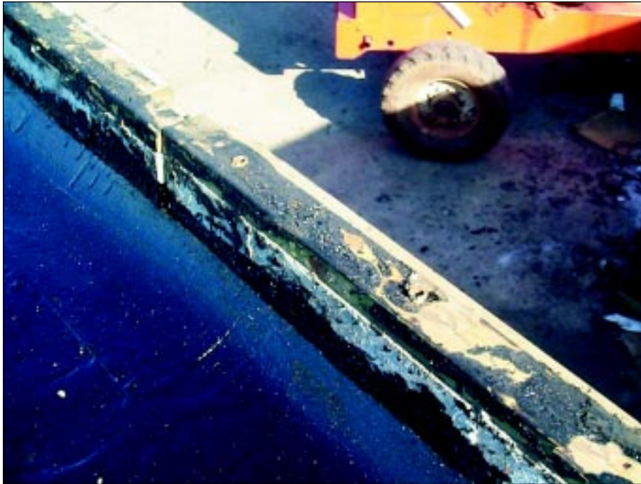
FIGURE 5-27: Nailer at the roof of the hospital in Stroud, Oklahoma. The roof surface in this photo was replaced prior to this photo, but the same nailer was used again during repairs.
