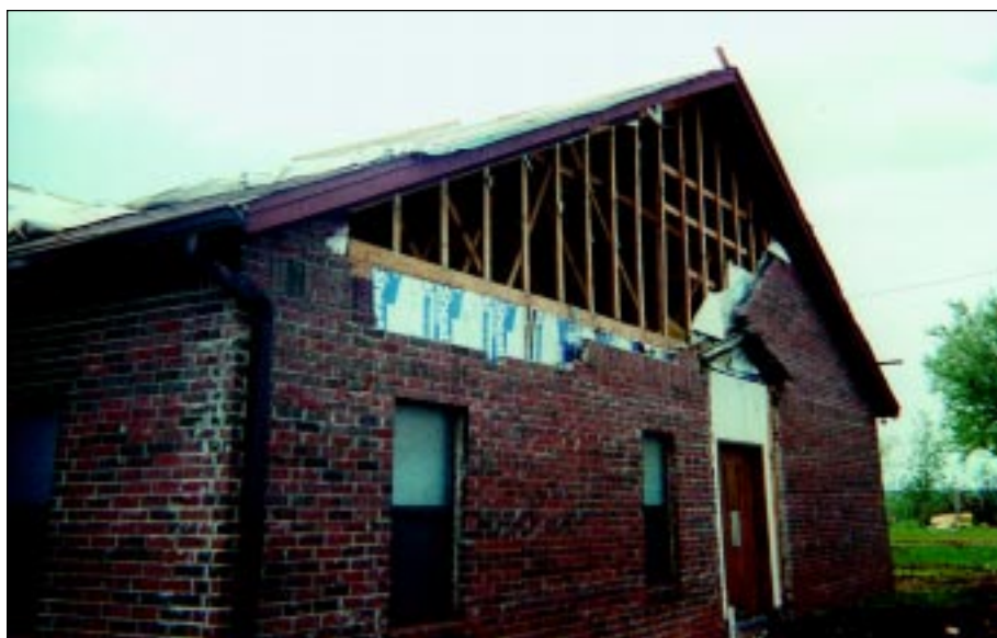
FIGURE 3-8: Failure of this gable wall section was due to wind suction forces on the leeward wall. This church was on the outer edge of a violent tornado path.
