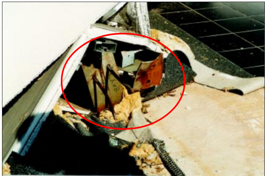
FIGURE 5-8: Column anchors that withdrew from concrete foundation at the regional outlet mall in Stroud, Oklahoma, hit by a strong tornado vortex.
