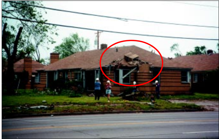
FIGURE 4-43: Chimney failure onto roof of single-family attached housing, Wichita, Kansas. This building was located along the periphery of a strong tornado.
