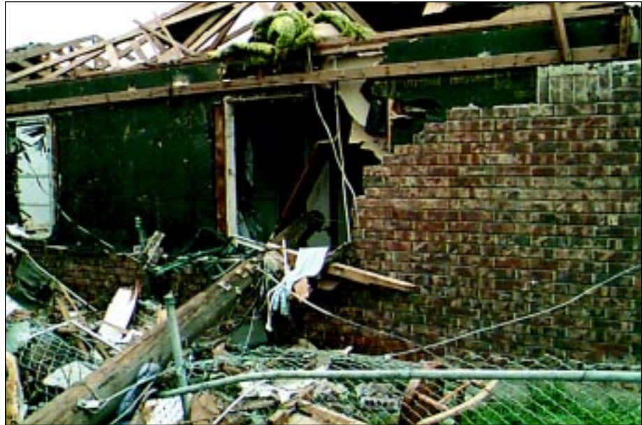
FIGURE 3-22: This power pole penetrated a window and extended several feet into the house after traveling approximately 40 feet from its original location. This home was located in Moore, Oklahoma, along the track of a violent tornado.
