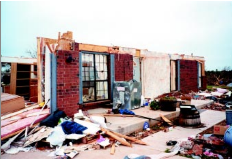
FIGURE 4-33: Brick veneer failure at the house shown in Figure 4-32.
