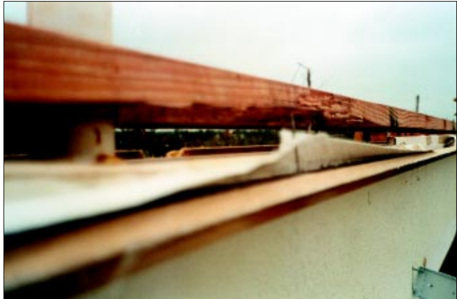
FIGURE 4-8: Failure of a double top-plate. The uplift of the roof truss previously attached to this double top-plate caused separation of the two members that comprise this top-plate.
