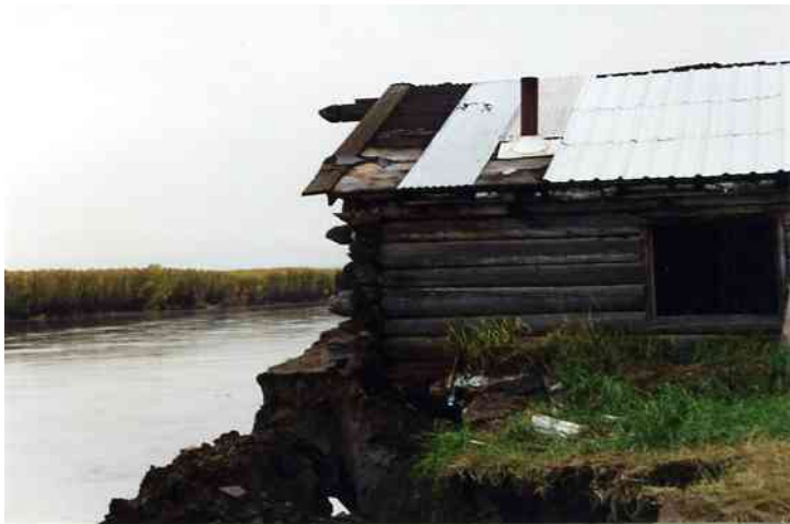
Photo 3: Log home undercut by erosion, 2004.
