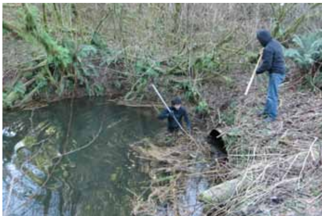
In preparation for installing a beaver deceiver (alternate dam site above the culvert), the existing plugged culvert is cleared.
