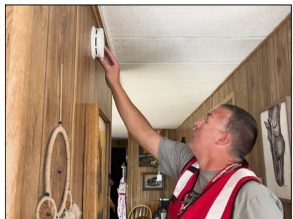
Rick Applegate installs a smoke alarm in a Meridian home. Teams installed 284 free alarms.
