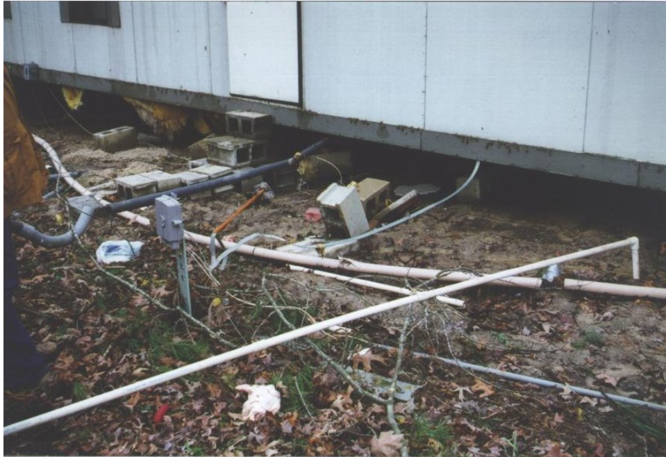
MHSW: DOD 3: Unit slides off block piers but remains upright
