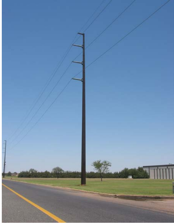
ETL: Single Steel Pole
