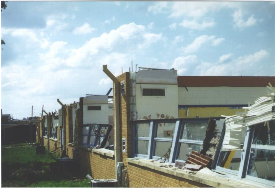
ES: DOD 7: Uplift of entire roof structure
