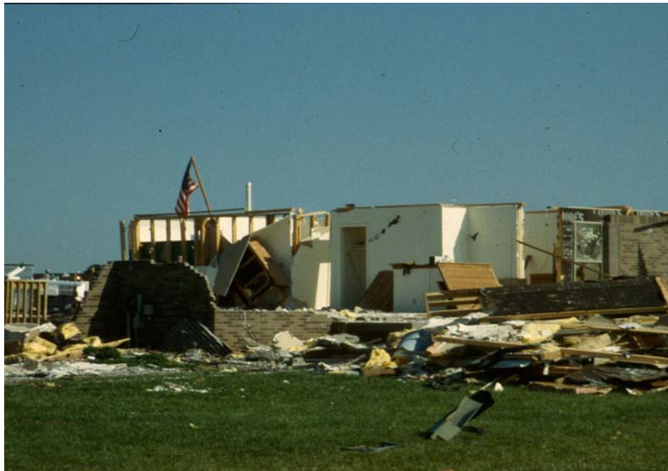
FR12: DOD 7: Top floor (First floor in this case) exterior walls collapsed
