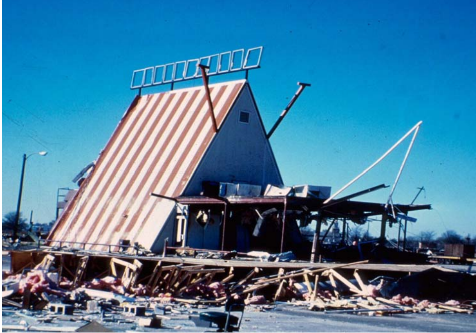
SRB: DOD 5: Canopies and covered walkways destroyed
