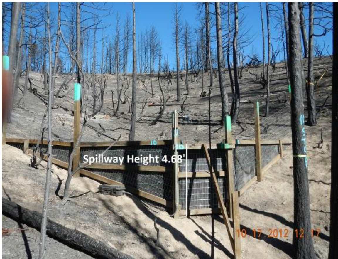
Figure ES-3. This photograph shows the upslope view at the back of a control site sediment fence. In this view both the sediment fence structure and most of the contributing swale can be seen. The spillway in the center of the fence is evident and the fence is braced with a post to counter the weight of captured sediment. Because it is a control site, this swale was not salvage-logged nor contour subsoiled and was disturbed only by the Ponderosa Fire itself. Note the relatively uniform nature of the soil surface which is covered by ash, the remnant dead trees evident throughout the burned swale and that there is no obvious stream channelization in the swale prior to the occurrence of post-wildfire rain. Although undisturbed by any post-wildfire treatment, the control sites produced the highest water runoff and average soil erosion during the over the first winter season (see Figures ES-7 and ES-8).
