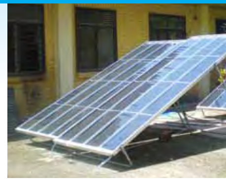
Solar panels used for water purification.
