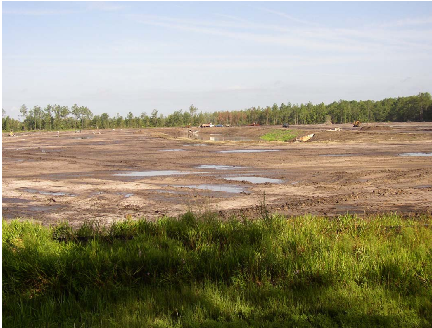
Building site with saturated soils on cleared forested wetlands, Glynn County. (Note filling on right.)
