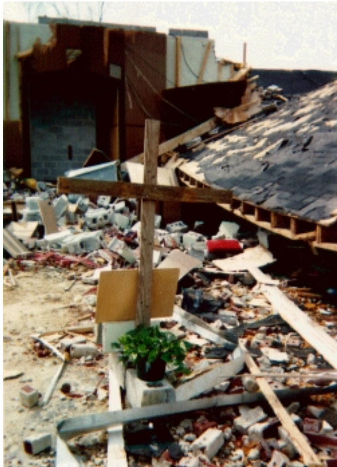
Two close-up views of the damaged inner sanctuary of the Goshen UMC. The collapsed roof is visible in both pictures. (Note, for orientation, see the cover photograph of the entire damaged church.) Photographs courtesy of Barry Reichenbaugh.
