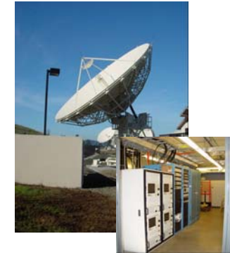
4 Signal Generator System/ Ground Earth Stations
