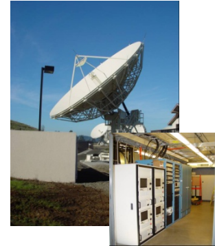
4 Ground Earth Stations
