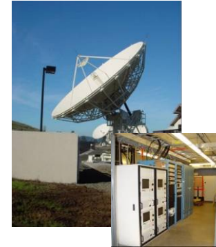
4 Ground Earth Stations
