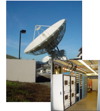
6 Ground Earth Stations
