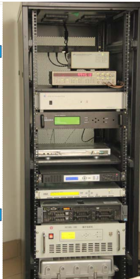
Equipments in Base Station
