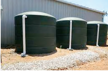
(Left) Rainwater cisterns in Pretoria, South Africa. PHOTO: USAID
