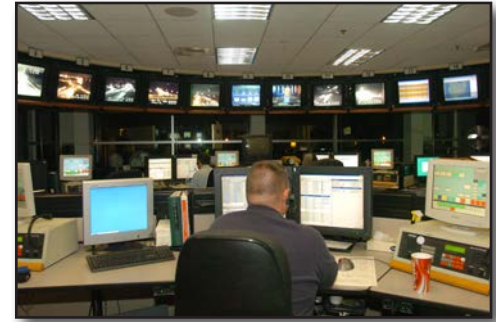
Figure 6.1 – Traffic control centers have myriad equipment used to monitor traffic and road conditions. (Photo/Bob Esposito, Pennsburg, Pennsylvania)
