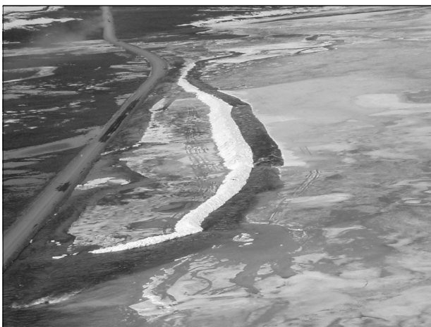
DOT built a snow dike to keep runoff from washing out the Dalton Hwy.
