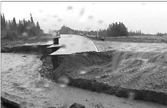
Richardson Hwy washed out south of Delta Junction
