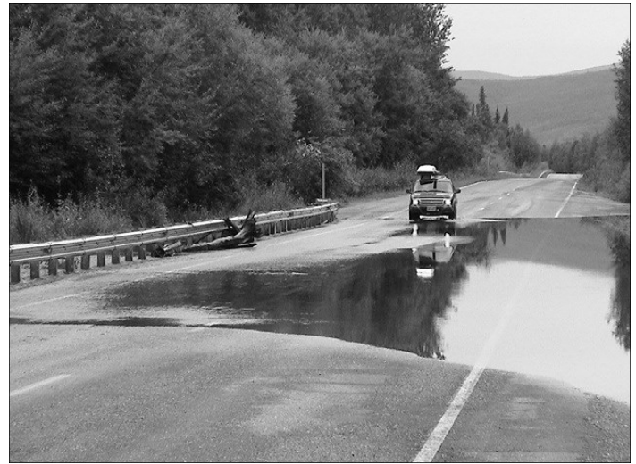
Minor flooding at Mile 31 of Chena Hot Springs Road in Fairbanks August 2003
