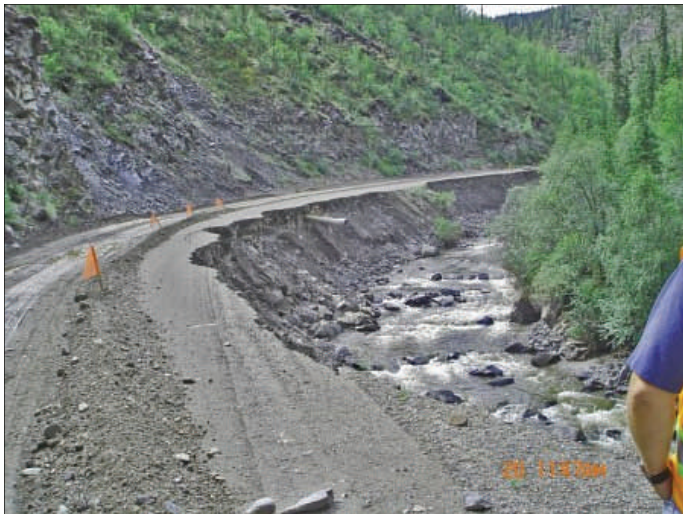
Taylor Highway at Milepost 152.8 and American Creek Between Mileposts 151 and 154 numerous sections of the highway washed out. This photo shows a loss of approximately 15 feet of roadway.
