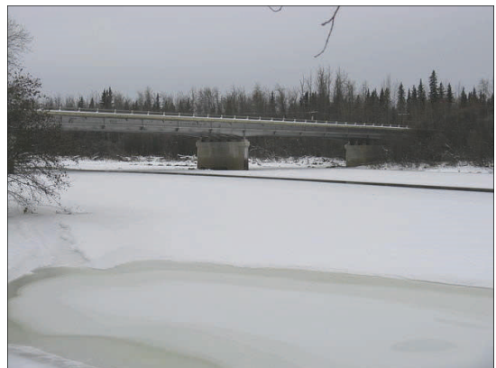
Freezeup at the Salcha River Bridge
