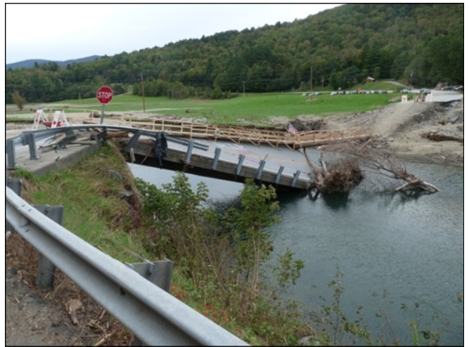
Bridge destroyed on Hwy 100 near Rochester, Vermont
