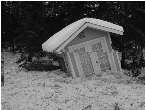
Damage to an outbuilding caused by the release of the Tazlina West glacier dammed lake Photo courtesy of local resident
