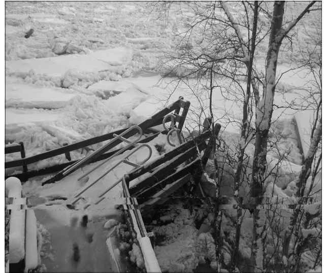
Damaged stairway at the Kenai River Center Photo courtesy of Kenai Peninsula Borough
