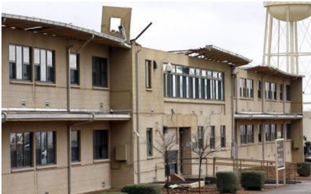
Damaged administrative building at White Sands Missile Range... Shari Vialpando Las Cruces Sun News
