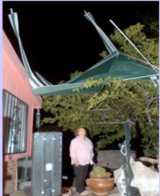
During the evening of Aug 28, thunderstorms produce wind gusts of almost 70 mph causing minor damage across Las Cruces. ( Photographed by Norm Dettlaff/Las Cruces Sun News)
