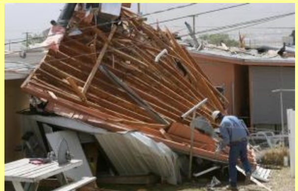
Wind gusts around 50 mph tear a roof from a building in El Paso on April 10. (Mark Lambie El Paso Times)
