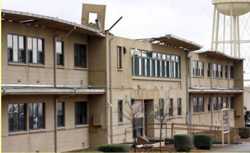
High winds seriously damaged the administrative building at White Sands Missile Range. (Shari Vialpando Las Cruces Sun News)
