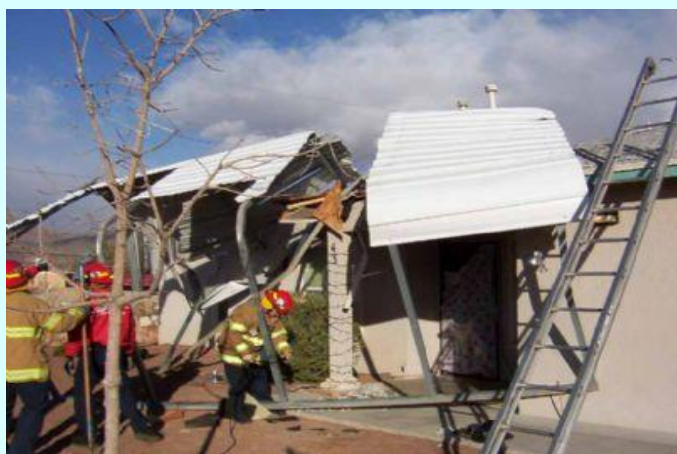
Winds blew down this carport in El Paso. (El Paso Fire Department for the El Paso Times)
